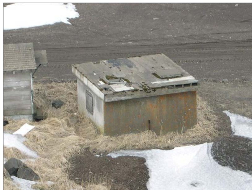
Winandy, David, photographer. 2006. Saltwater Well House 1, March 21, 2006. Photograph (digital) . NOAA, NOS, Pribilof Project Office, Seattle.
