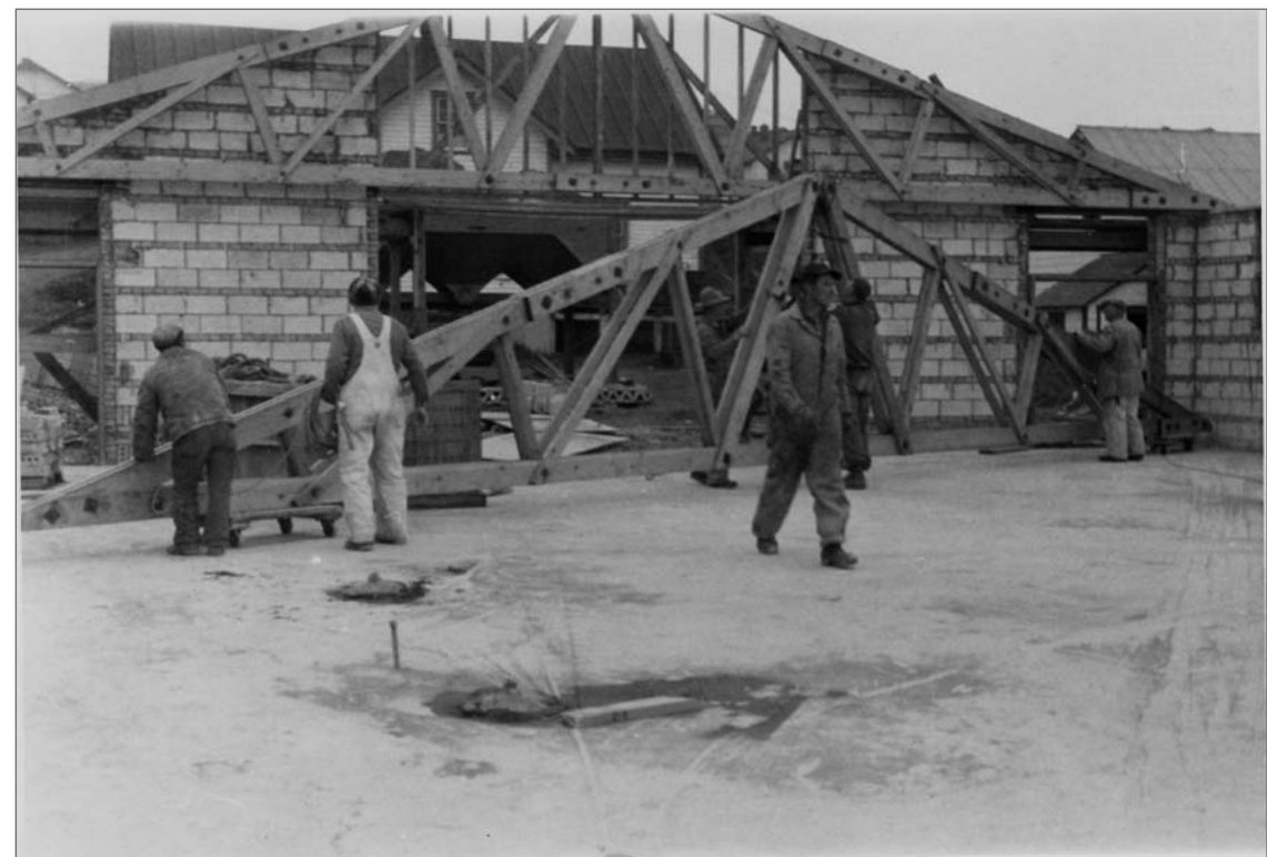
Photograph No. 95-ADMC-1993 (Photographer unknown), 1950's; Men installing trusses, Community Store/Warehouse/Laboratory, looking west. Records of the National Oceanic and Atmospheric Administration, RG 370; NARA—Pacific Alaska Region (A).
