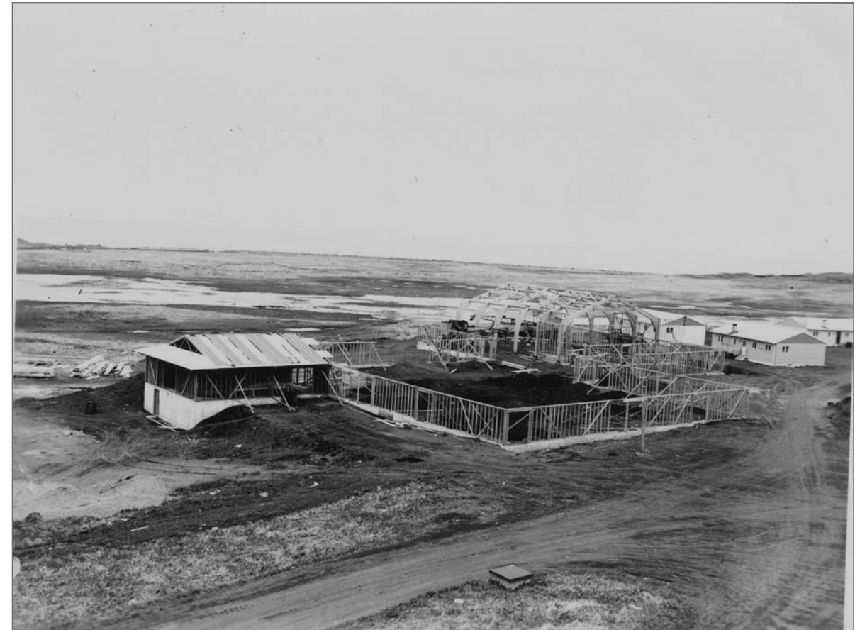
Photograph No. 95-ADMC-2173 (Photographer unknown), 1972; Construction of St. Paul Elementary and Junior High School. Records of the National Oceanic and Atmospheric Administration, RG 370; NARA—Pacific Alaska Region (A).
