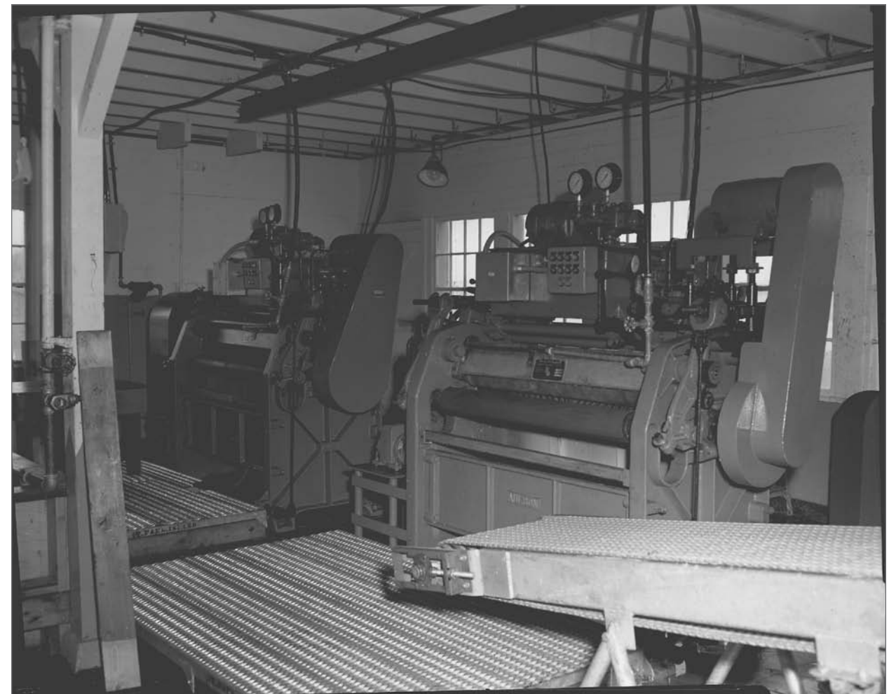
Photograph No. 95-ADMC-1476; (Photographer unknown), 1972; Interior, By-Products Plant showing conveyor belt and machinery. Records of the National Oceanic and Atmospheric Administration, RG 370; NARA—Pacific Alaska Region (A).
