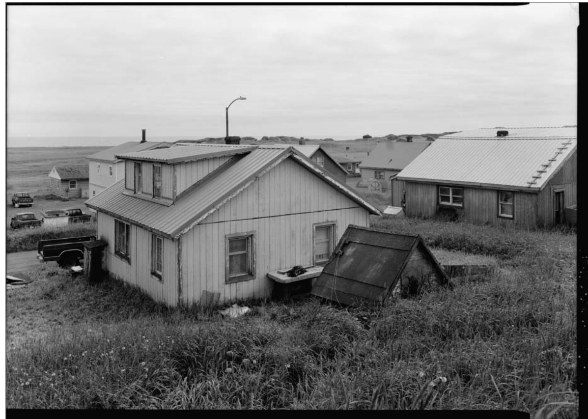
North and west sides, House 49. Jet Lowe, photographer. Photograph (5x7) . Library of Congress: HABS AK-203-2 , 2004.
