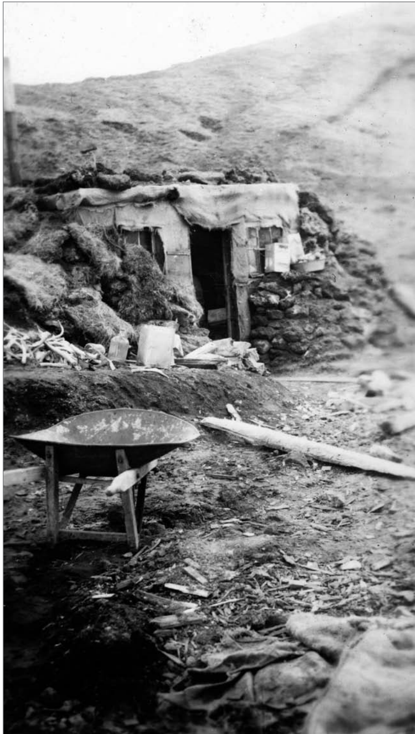
Hill, Evan, photographer. 1943. U.S. Army observation post under construction on hillside. Note: These dugouts are not barabaras. Photograph. Alaska State Library, Historical Collections: PCA 343, Evan Hill Photograph Collection, P343.415.
