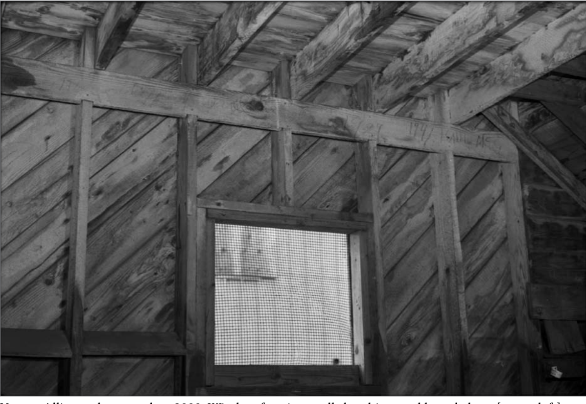
Young, Allison, photographer. 2000. Window framing, wall sheathing, and barrel chute [upper left], northwest wall interior, 1st floor Salthouse A. Photograph (35mm). NOAA, NOS, Pribilof Project Office, Seattle: sheet JL 110929.4, neg. 3982.
