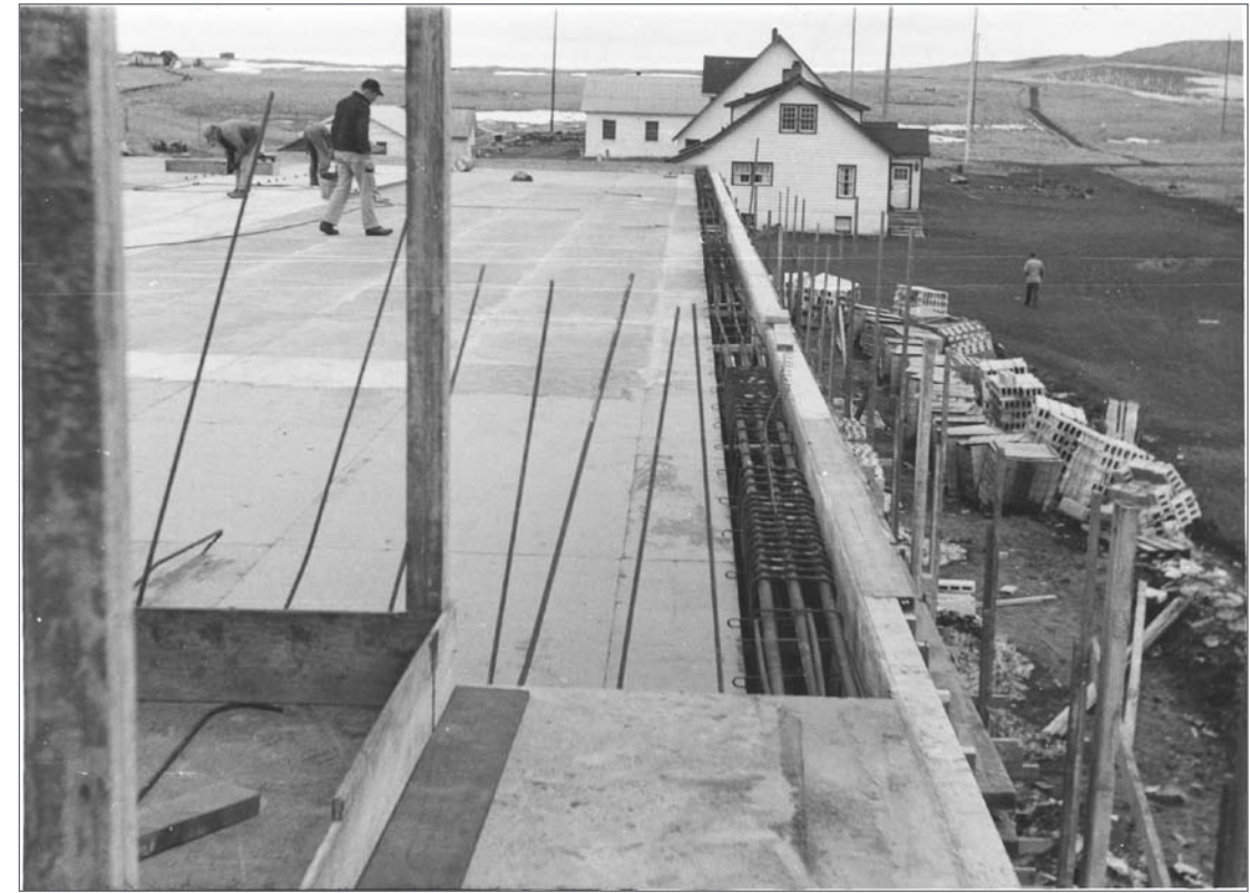
Photograph No. 95-ADMC-2035 (Photographer unknown), 1950's; Community Store/Warehouse/Laboratory under construction, looking east. Records of the National Oceanic and Atmospheric Administration, RG 370; NARA—Pacific Alaska Region (A).
