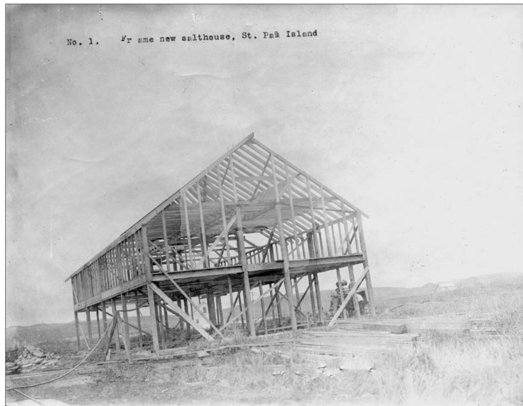
Photograph No. 22-MP-3-74 (Photographer unknown), 1919; New Salthouse under construction. In 1910, there were five salthouses on St. Paul Island, one at Northeast Point, one at Rocky Point, one called the Cove Salthouse situated at the northeast end of the Village Cove, a large Village Salthouse, and a small building opposite it that was used for storage of new salt. The small building was moved to serve as a hospital in 1914. The Rocky Point and Cove Salthouses were razed before 1919. Records of the National Oceanic and Atmospheric Administration, RG 370; NARA—Pacific Alaska Region (A).
