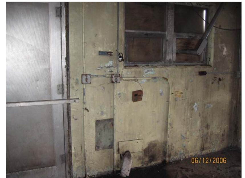
Barnea, Nir, photographer. June 12, 2006. Interior, former Power Plant. Photograph (digital). NOAA, NOS, Pribilof Project Office, Seattle.
