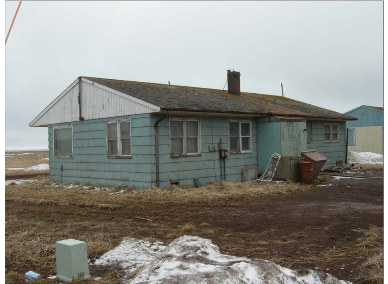
Mobley, Charles, photographer. 2007. North and west sides, Aleut Laborer House 127. Photograph (35mm). NOAA, NOS, Pribilof Project Office, Seattle.
