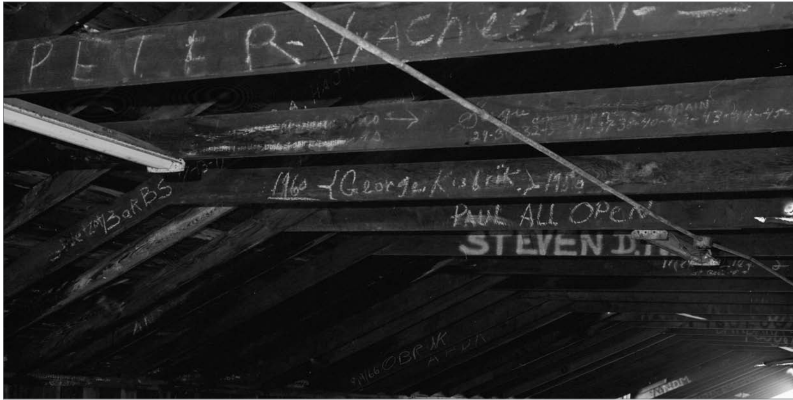
Lindsay, John A., photographer. 2000. Graffiti on ceiling rafters and cross braces; second floor of Salthouse A. Photograph (6x7cm) . NOAA, NOS, Pribilof Project Office, Seattle: JL111381.10, neg. 3864.
