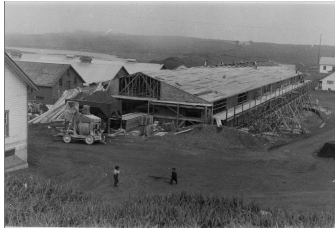
Photograph No. 95-ADMC-1998 (Photographer unknown), 1950's; Installing roof, Community Store/Warehouse/Laboratory under construction, looking east northeast. Records of the National Oceanic and Atmospheric Administration, RG 370; NARA—Pacific Alaska Region (A).
