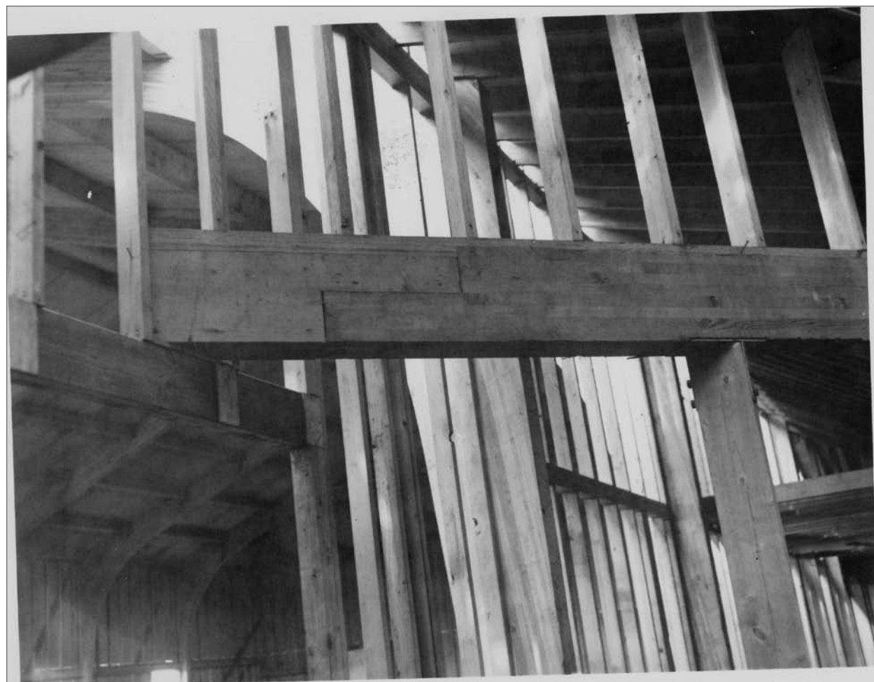
Photograph No. 95-ADMC-2169 (Photographer unknown), July 31, 1972; Construction of St. Paul Elementary and Junior High School. Records of the National Oceanic and Atmospheric Administration, RG 370; NARA—Pacific Alaska Region (A).
