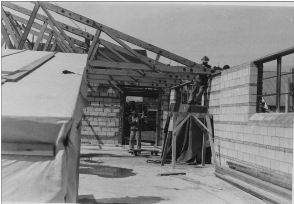
Photograph No. 95-ADMC-2000 (Photographer unknown), 1950's; Men installing trusses, Community Store/Warehouse/Laboratory, looking west. Records of the National Oceanic and Atmospheric Administration, RG 370; NARA—Pacific Alaska Region (A).
