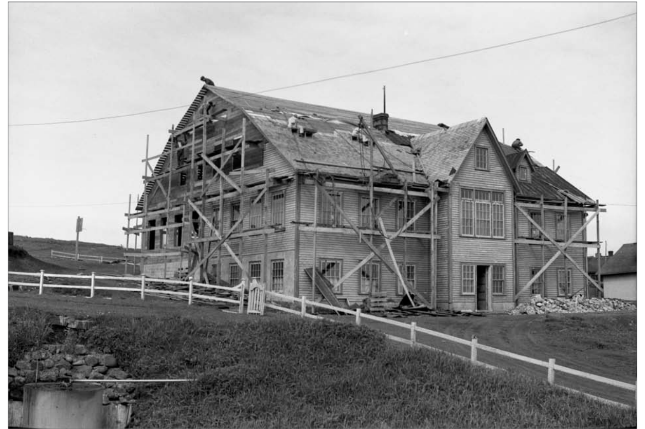
Photograph No. 22-RB-1949-14 (Photographer unknown), 1949; School addition under construction, St. Paul Island, Alaska. Records of the U.S. Fish and Wildlife Service, RG 22; NARA, Special Media Archives Services Division, National Archives at College Park, College Park, MD.
