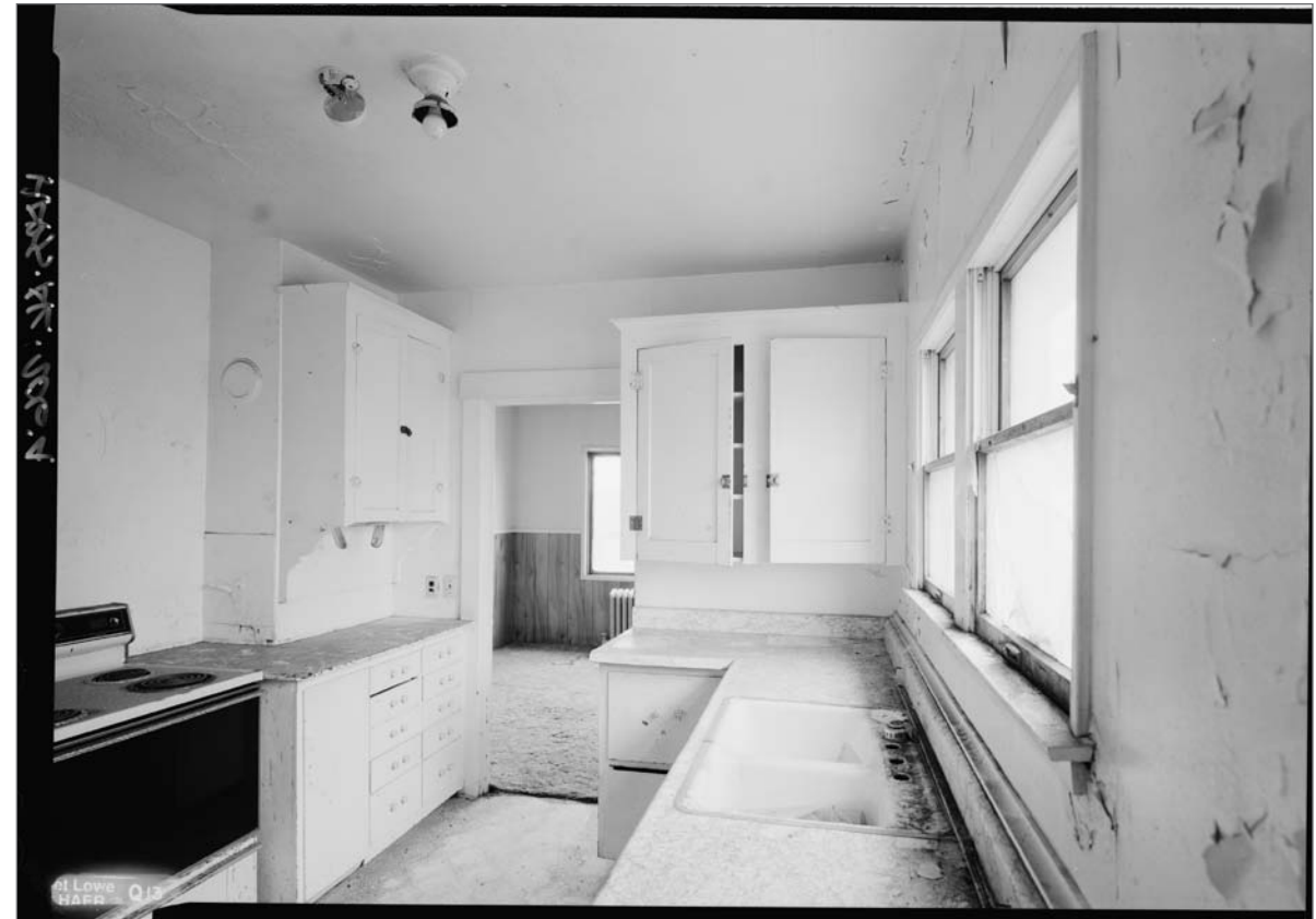
Interior, Teacher House 101, looking from kitchen to dining room (West to East). Jet Lowe, photographer. Photograph (5x7). Library of Congress: HABS AK-206-4, 2004.
