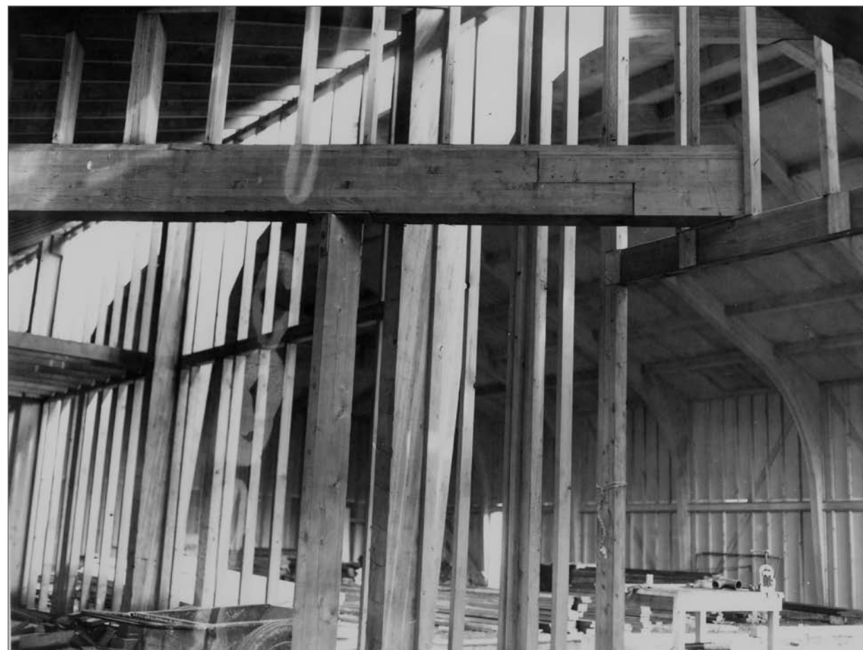
Photograph No. 95-ADMC-2174 (Photographer unknown), July 31, 1972; Construction of St. Paul Elementary and Junior High School. Records of the National Oceanic and Atmospheric Administration, RG 370; NARA—Pacific Alaska Region (A).
