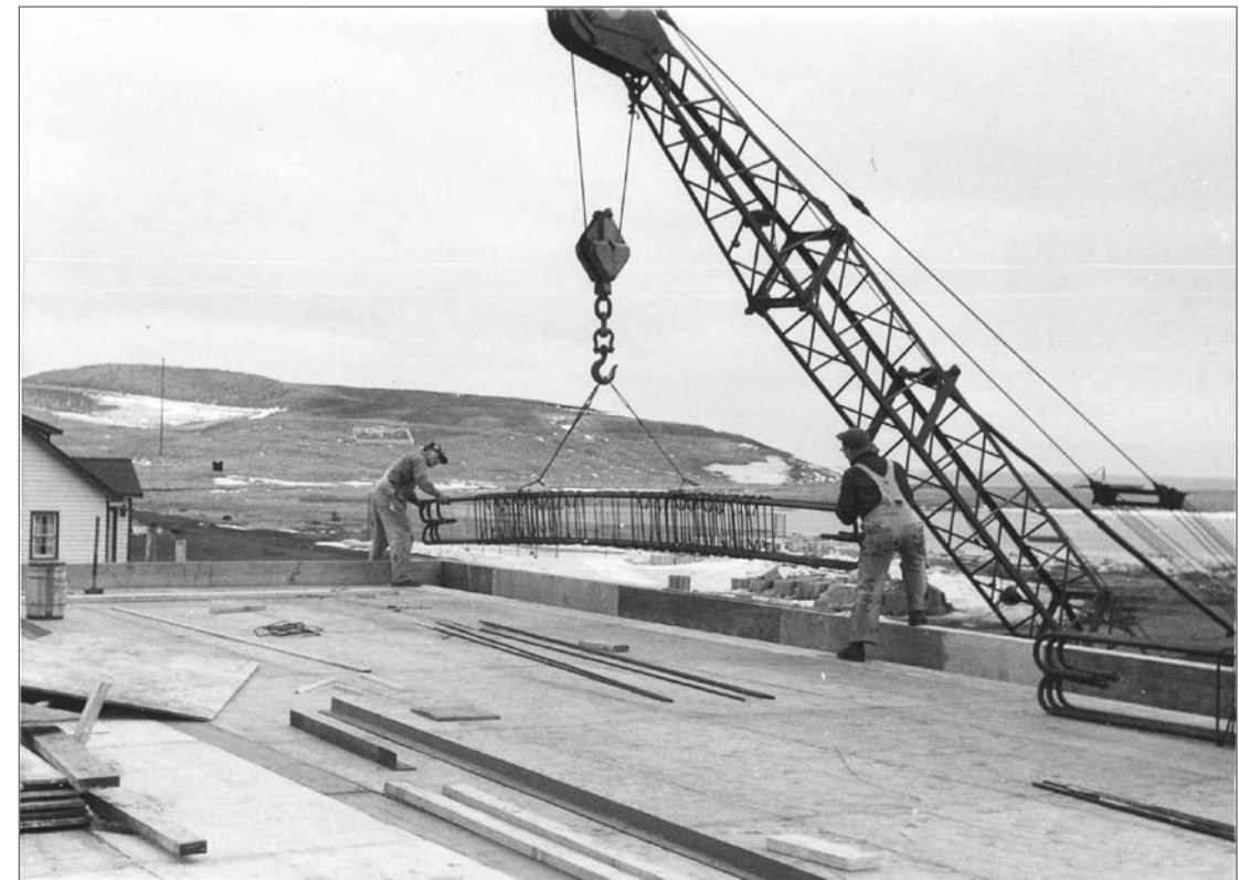
Photograph No. 95-ADMC-2024 (Photographer unknown), 1950's; Community Store/Warehouse/Laboratory under construction, looking east. Records of the National Oceanic and Atmospheric Administration, RG 370; NARA—Pacific Alaska Region (A).
