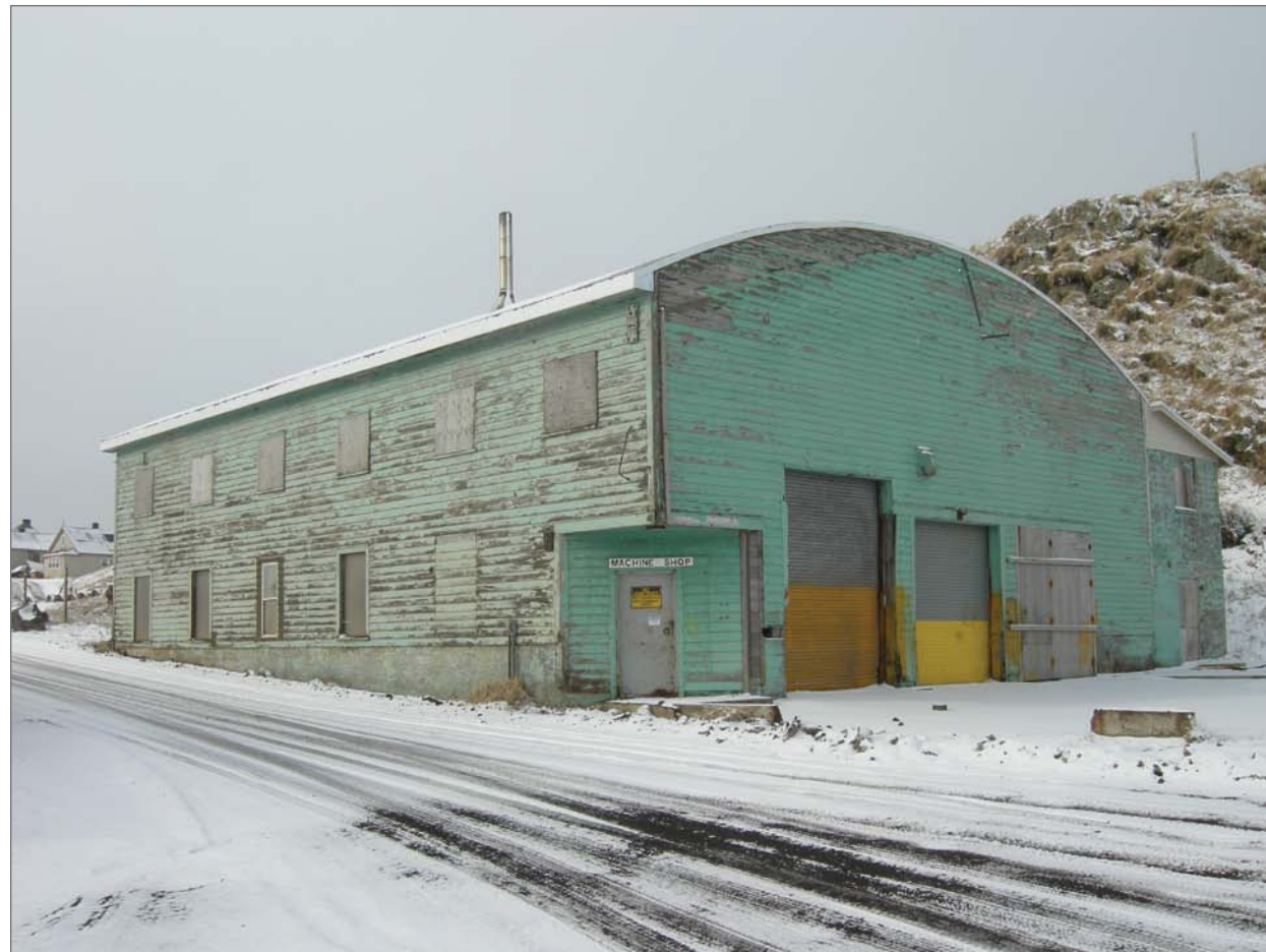
Mobley, Charles, photographer. 2007. East side and north front, Machine Shop. Photograph (35mm) . NOAA, NOS, Pribilof Project Office, Seattle.
