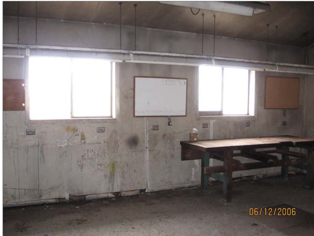
Barnea, Nir, photographer. June 12, 2006. Interior, former Power Plant. Photograph (digital) . NOAA, NOS, Pribilof Project Office, Seattle.
