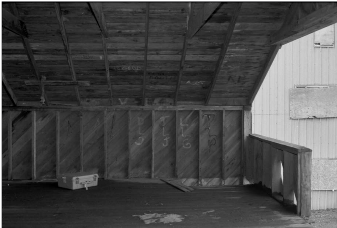
Young, Allison, photographer. 2000. Salthouse A, 2nd floor interior, west wall (north to south: left to right), Fouke Bunkhouse in far right view. Photograph (35mm). NOAA, NOS, Pribilof Project Office, Seattle: sheet JL 111379.4, neg. 4191; series includes negatives 4191 through 4202, excluding 4195.
