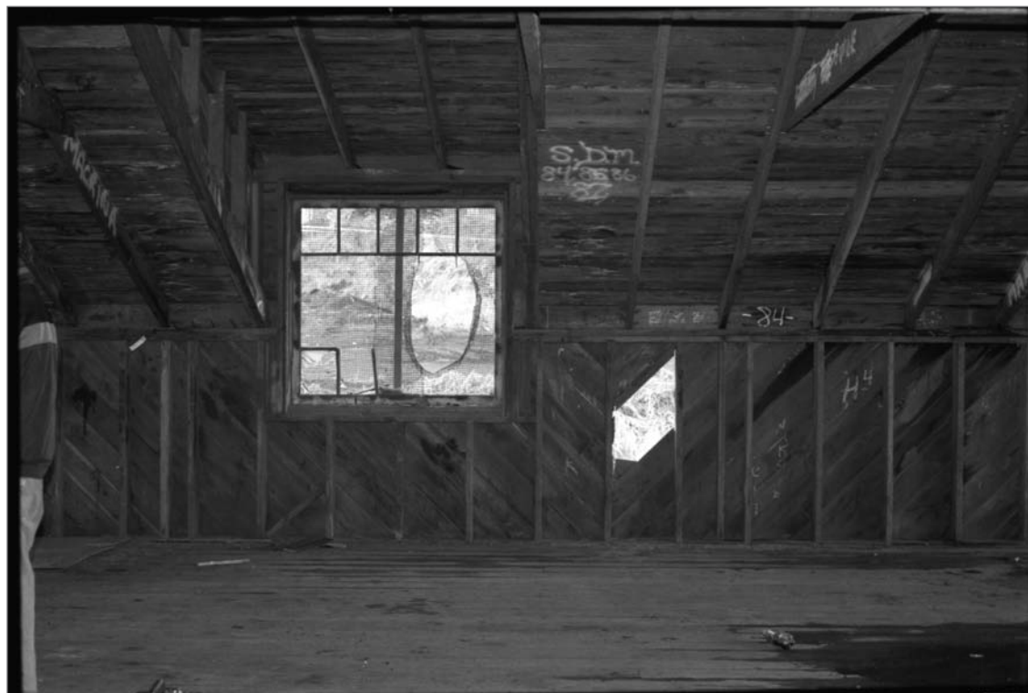
Young, Allison, photographer. 2000. Salthouse A, 2nd floor interior, west wall (north to south: left to right). Note rope linked with the building structure was used to pull the building down. Photograph (35mm). NOAA, NOS, Pribilof Project Office, Seattle: sheet JL 111379.4, neg. 4194, NMML; series includes negatives 4191 through 4202, excluding 4195.
