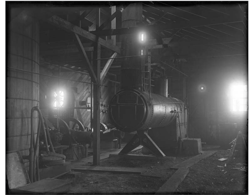
Photograph No. USBF 1.42 (Photographer G Dallas Hanna), 1919; Boiler providing steam power in By-Products Plant. Records of the National Oceanic and Atmospheric Administration, RG 370; NARA—Pacific Alaska Region (A).
