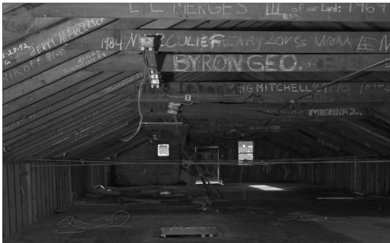
Lindsay, John A., photographer. 2000. Graffiti on ceiling rafters and cross braces; looking north on the second floor of Salthouse A. Photograph (6x7cm). NOAA, NOS, Pribilof Project Office, Seattle: sheet JL110930.5, neg. 4373.
