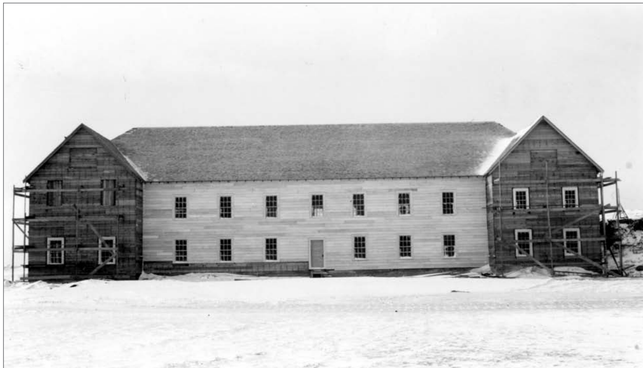
Olson, Clarence L., photographer. Circa 1951. East and north sides, Recreation Hall, under construction. Photograph . Courtesy Clarence L. Olson Collection; Anchorage Museum, B90-8-34.
