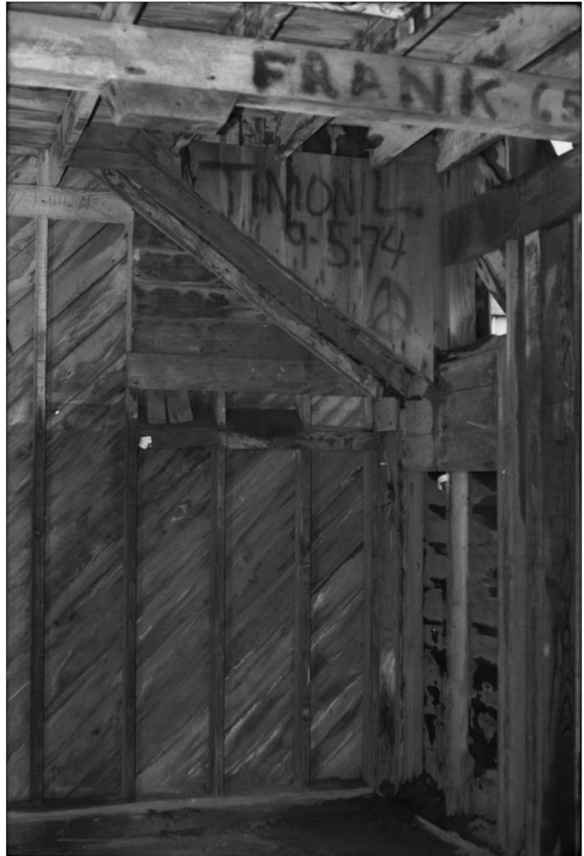
Young, Allison, photographer. 2000. Paint "Frank 65" on ceiling rafter; Paint "Timon L. 9-5-74" and peace symbol on barrel chute sheathing, northwest wall interior, 1st floor Salthouse A. Photograph (35mm). NOAA, NOS, Pribilof Project Office, Seattle: sheet JL 110929.4, neg. 3977.
