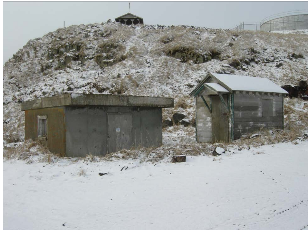
Mobley, Charles, photographer. 2007. Concrete Pump House. Photograph (35mm) . NOAA, NOS, Pribilof Project Office, Seattle.
