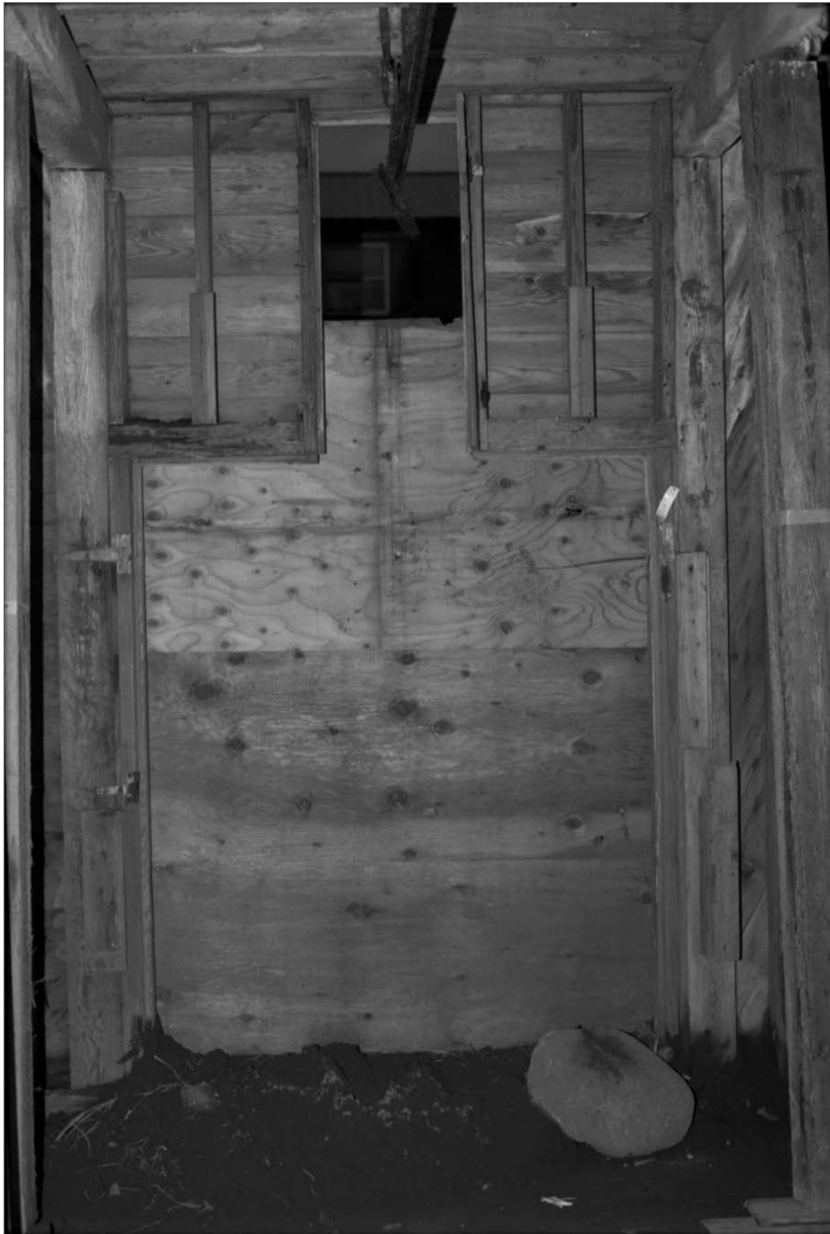
Young, Allison, photographer. 2000. Salthouse A, interior view, south end, Key-Hole door (boarded up) with overhead crane rail, benches on left and right forward of the door. Photograph (35mm). NOAA, NOS, Pribilof Project Office, Seattle: sheet JL 110929.3, neg. 4122.
