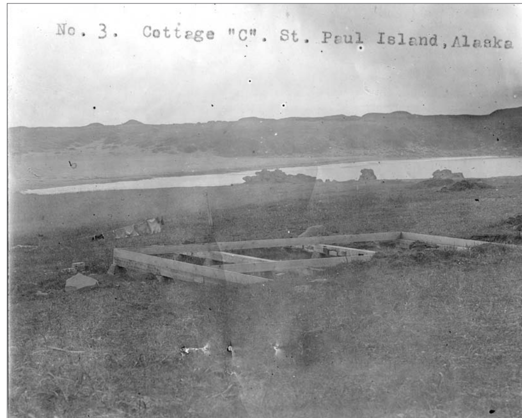
Photograph No. 22-MP-3-56 (Photographer unknown), circa 1919; Cottage "C" under construction, looking south southeast. RG 370; NARA—Pacific Alaska Region (A).
