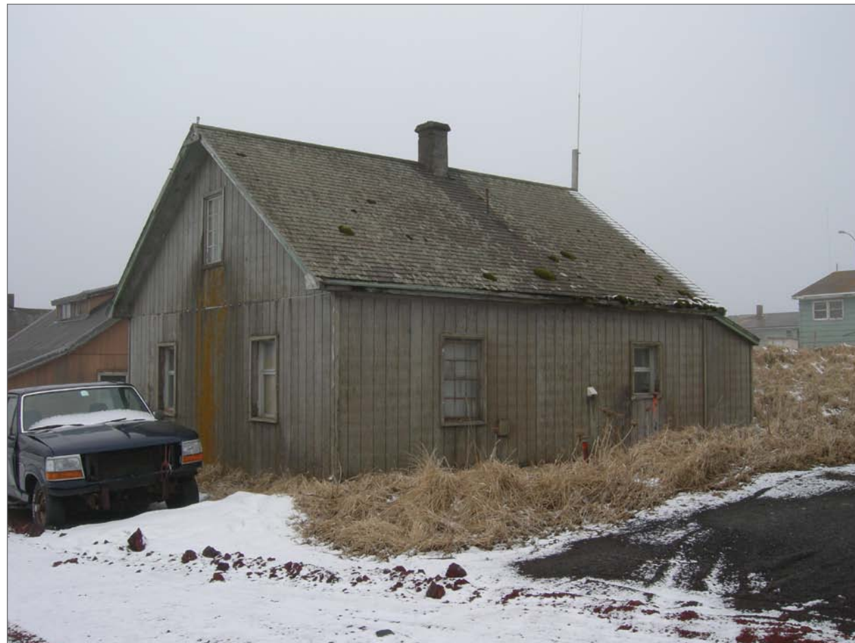
Mobley, Charles, photographer. 2007. East and north sides, Aleut Laborer House 26. Photograph (35mm). NOAA, NOS, Pribilof Project Office, Seattle.
