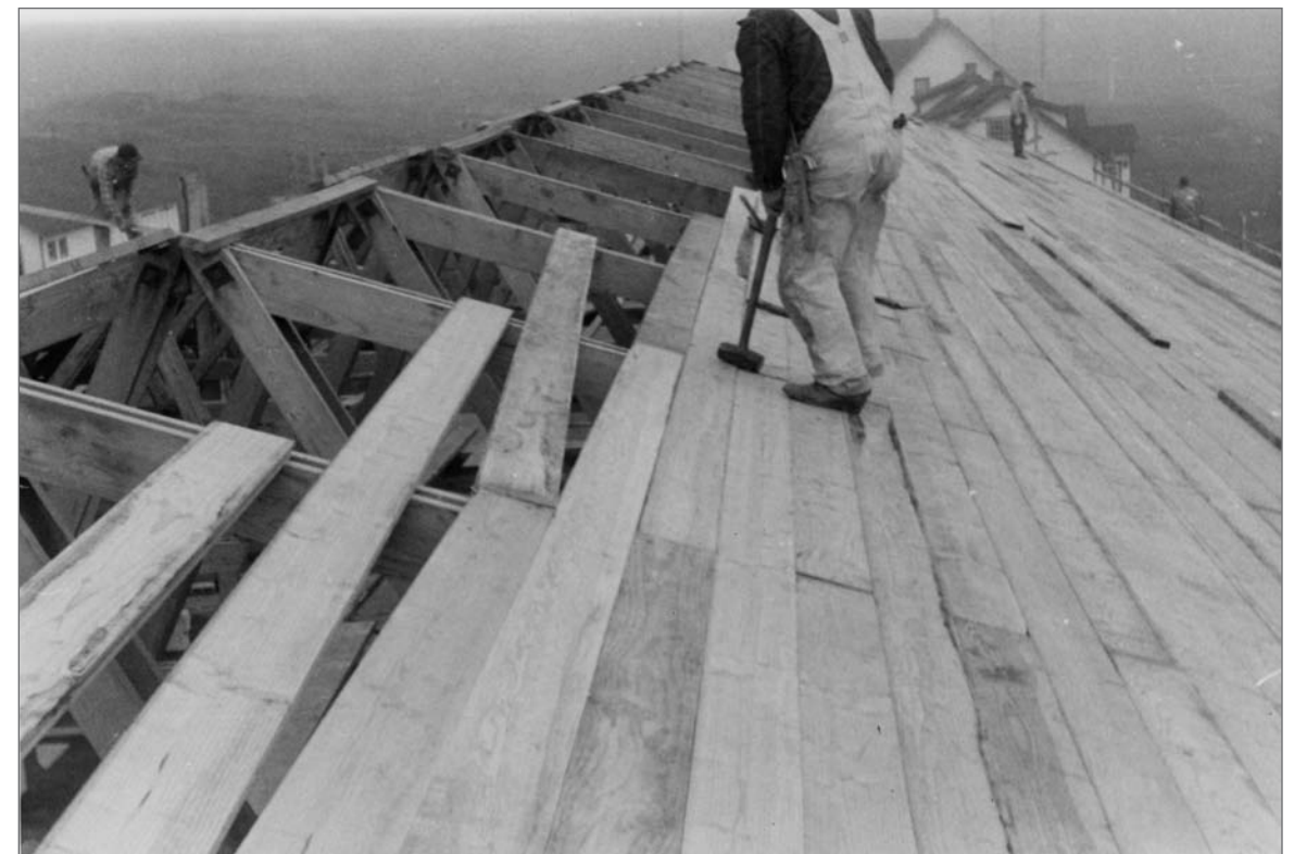
Photograph No. 95-ADMC-2004 (Photographer unknown), 1950's; Installing roof, Community Store/Warehouse/Laboratory under construction, looking east. Records of the National Oceanic and Atmospheric Administration, RG 370; NARA—Pacific Alaska Region (A).
