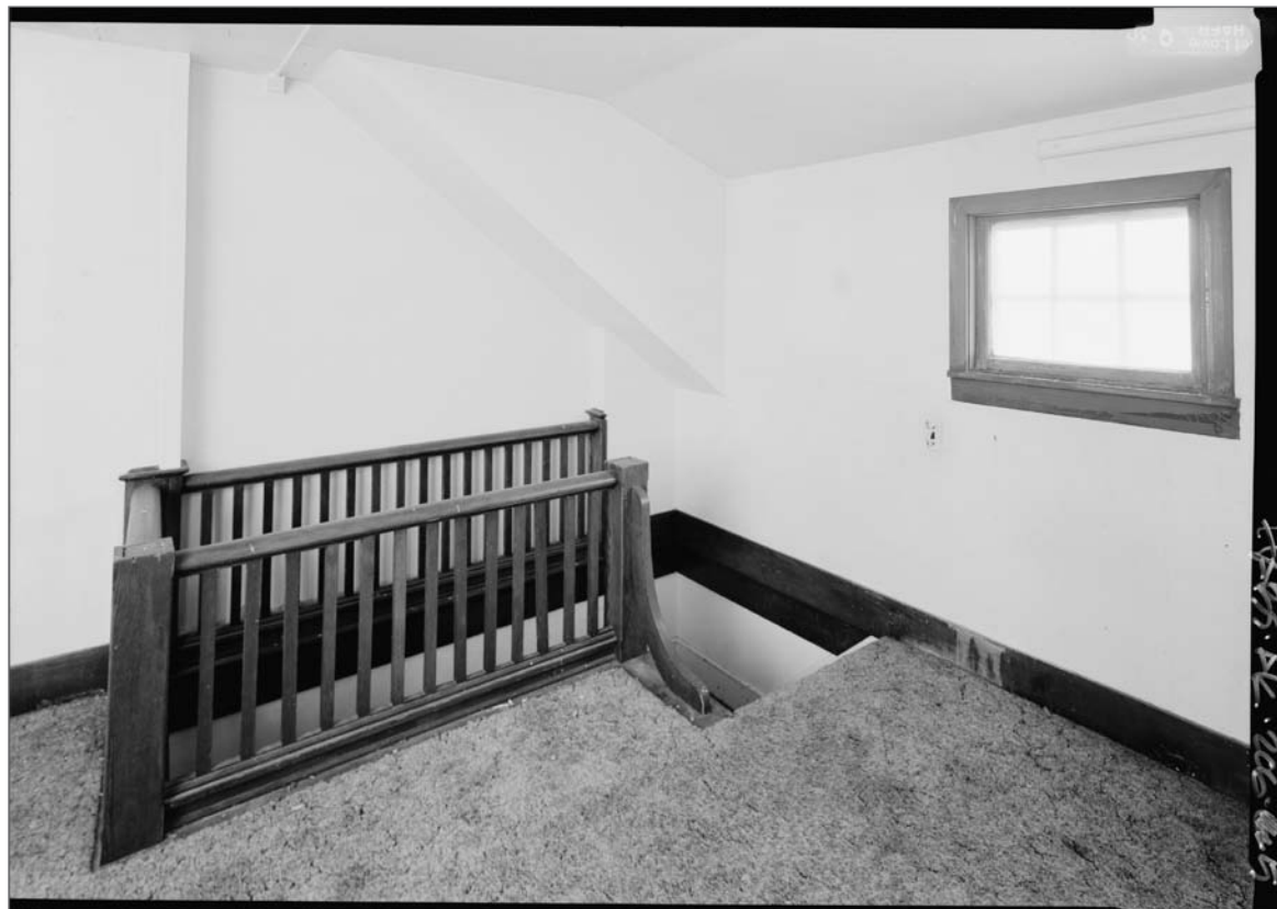
Interior, Teacher House 101, stair opening at second floor (window on West side). Jet Lowe, photographer. Photograph (5x7). Library of Congress: HABS AK-206-5, 2004.
