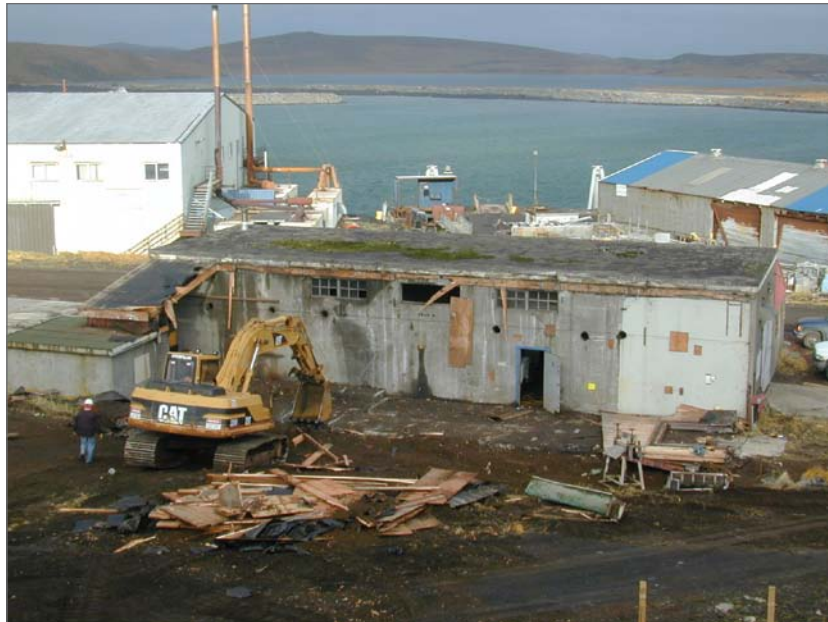
Photographer unknown. 2002. East and south sides, former Power Plant. Photograph (digital). NOAA, NOS, Pribilof Project Office, Seattle.
