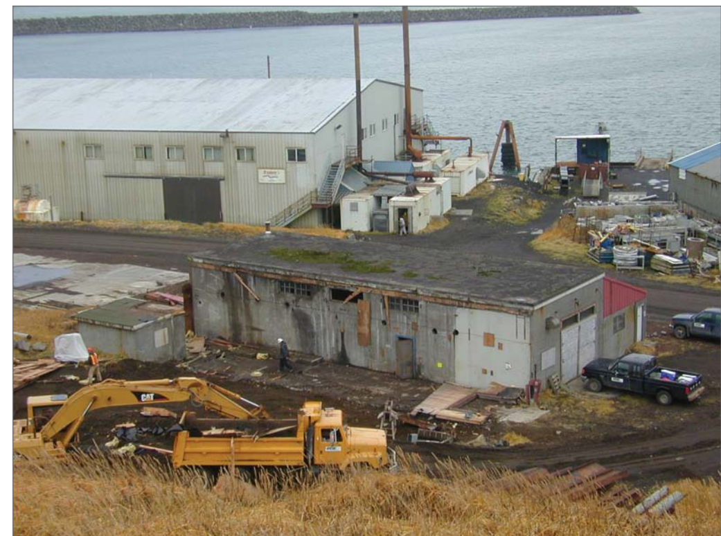
Photographer unknown. 2002. East and south sides, former Power Plant. Photograph (digital) . NOAA, NOS, Pribilof Project Office, Seattle.
