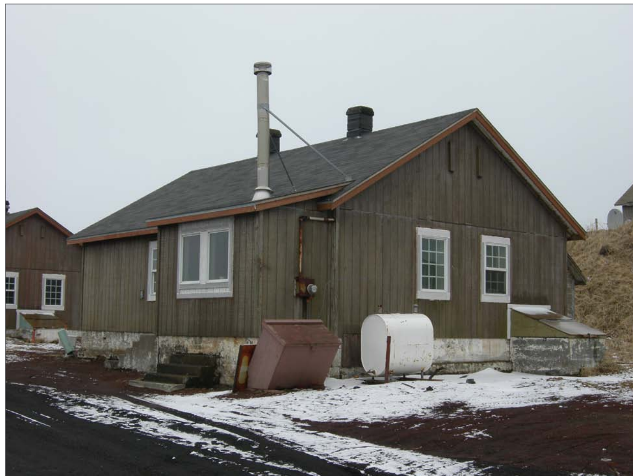
Mobley, Charles, photographer. 2007. East front and north side, Aleut Laborer House 38. Photograph (35mm). NOAA, NOS, Pribilof Project Office, Seattle.
