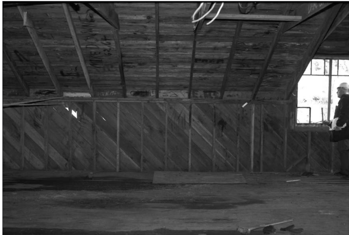
Young, Allison, photographer. 2000. Salthouse A, 2nd floor interior, west wall (north to south: left to right). Note rope (far left) linked with the building structure was used to pull the building down. Photograph (35mm). NOAA, NOS, Pribilof Project Office, Seattle: sheet JL 111379.4, neg. 4196, NMML; series includes negatives 4191 through 4202, excluding 4195.
