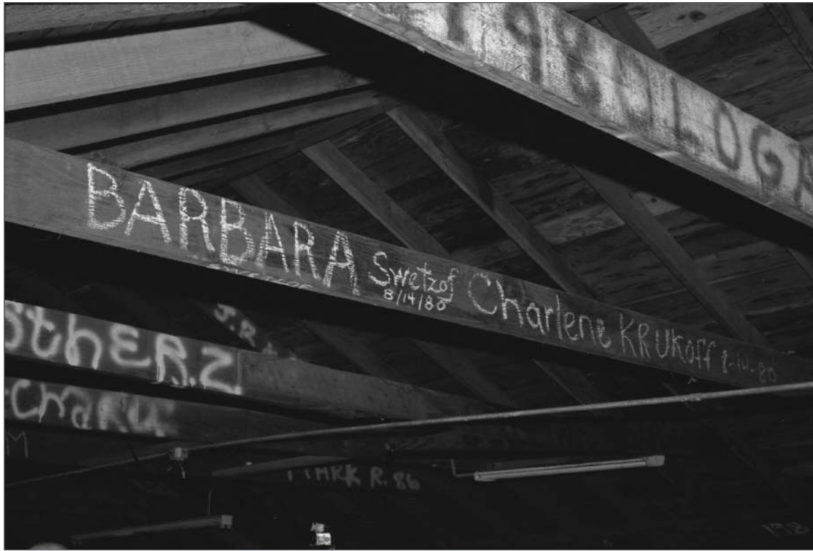
Young, Allison, photographer. 2000. Chalk "Barbara Swetzo 8-14-80, Charlene Krukoff 8-14-80" on joist, 2nd floor Salthouse A. Photograph (35mm). NOAA, NOS, Pribilof Project Office, Seattle: sheet JL 110929.2, neg. 4063.
