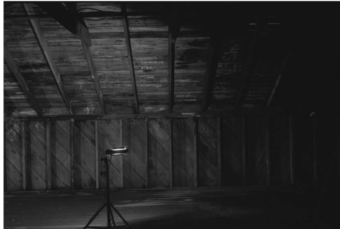
Young, Allison, photographer. 2000. Salthouse A, 2nd floor interior, west wall (north to south: left to right), photographer's TOTA lamp with stand on floor. Photograph (35mm). NOAA, NOS, Pribilof Project Office, Seattle: sheet JL 111379.4, neg. 4201, NMML; series includes negatives 4191 through 4202, excluding 4195.
