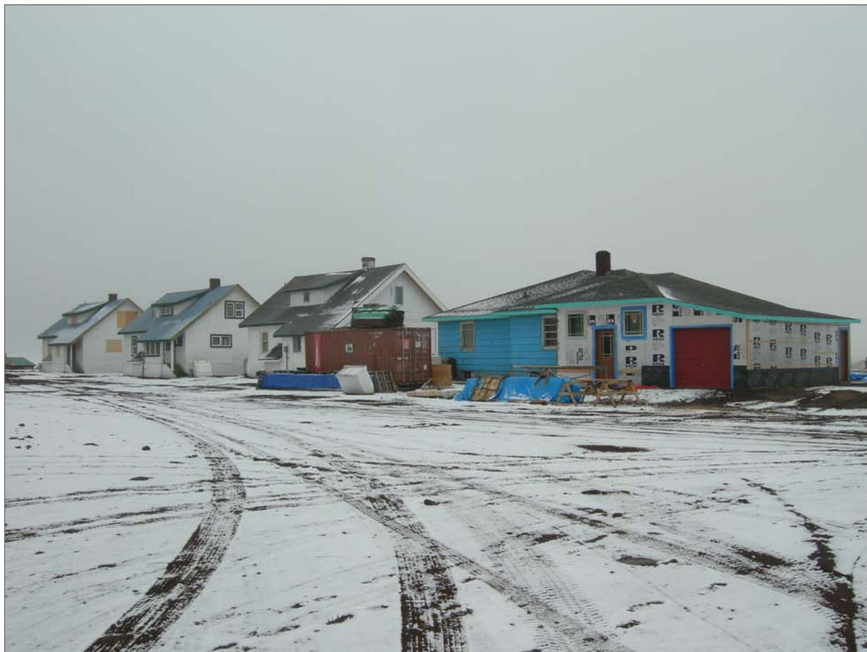
Mobley, Charles, photographer. 2007. Manager's House/House 115, undergoing a re-model, looking north-east, showing Teacher Houses to the left. Photograph (35mm) . NOAA, NOS, Pribilof Project Office, Seattle.
