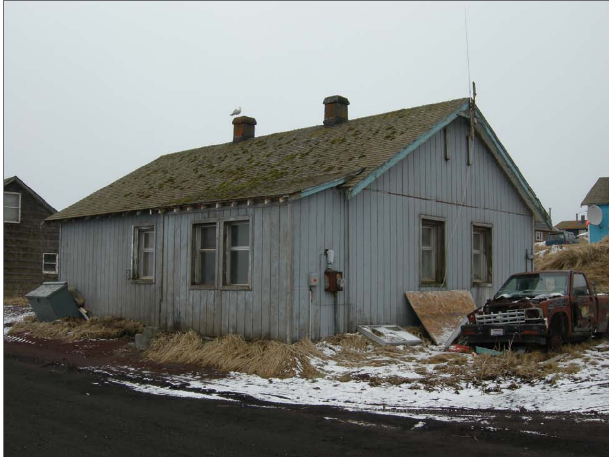
Mobley, Charles, photographer. 2007. East front and north side, Aleut Laborer House 40. Photograph (35mm). NOAA, NOS, Pribilof Project Office, Seattle.
