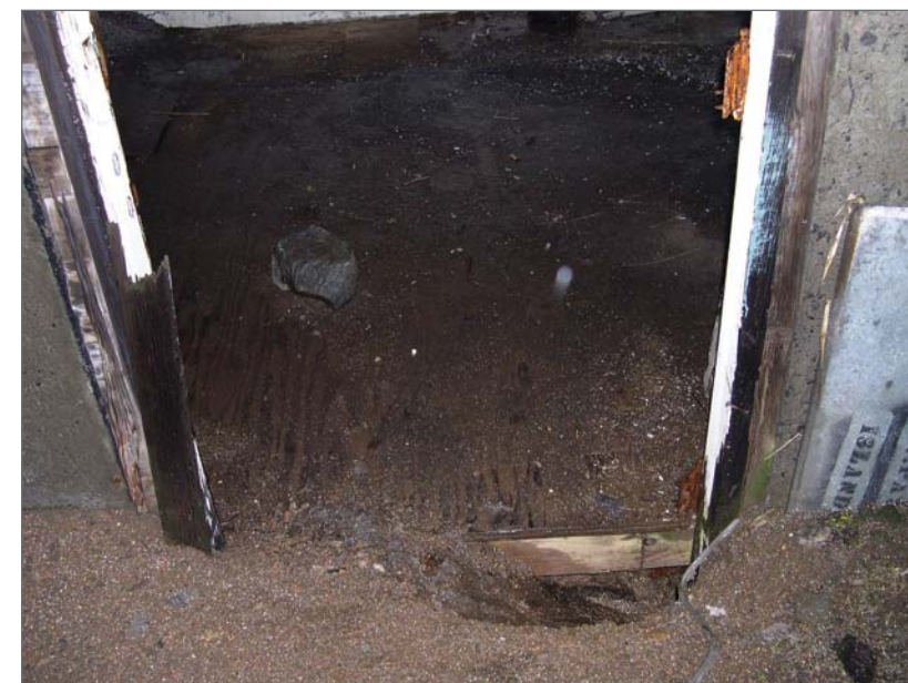
Winandy, David, photographer. 2006. Interior, Saltwater Well House 3, March 21, 2006. Photograph (digital) . NOAA, NOS, Pribilof Project Office, Seattle.
