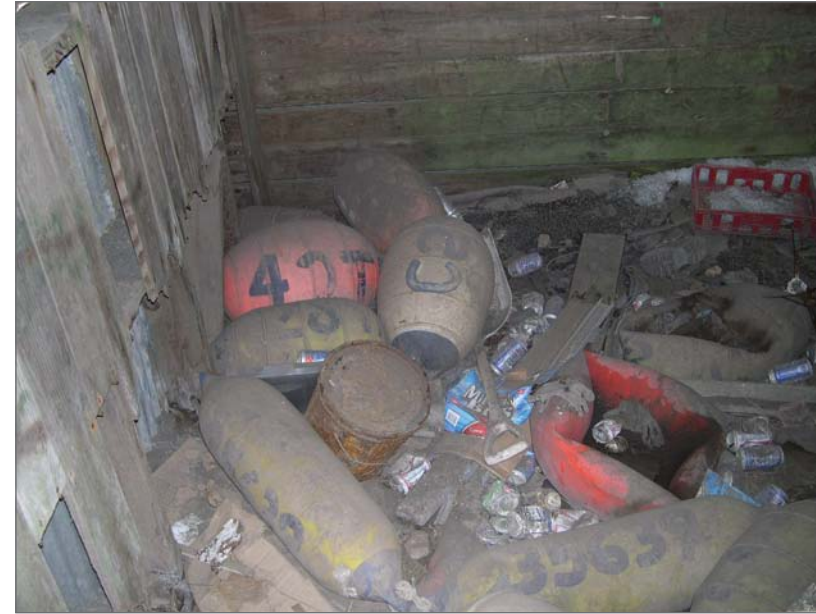
Winandy, David B., photographer. March 21, 2006. Interior, Shingle Shed, with crab pot buoy and other debris. Photograph (digital). NOAA, NOS, Pribilof Project Office, Seattle.
