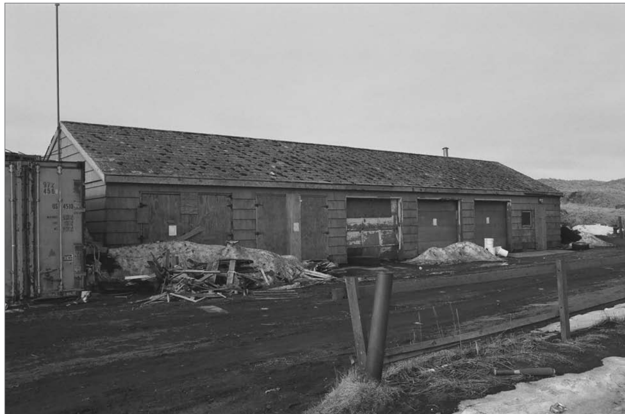
Mobley, Charles, photographer. 2007. West side and south front, Five-Car Garage. Photograph (35mm) . NOAA, NOS, Pribilof Project Office, Seattle.
