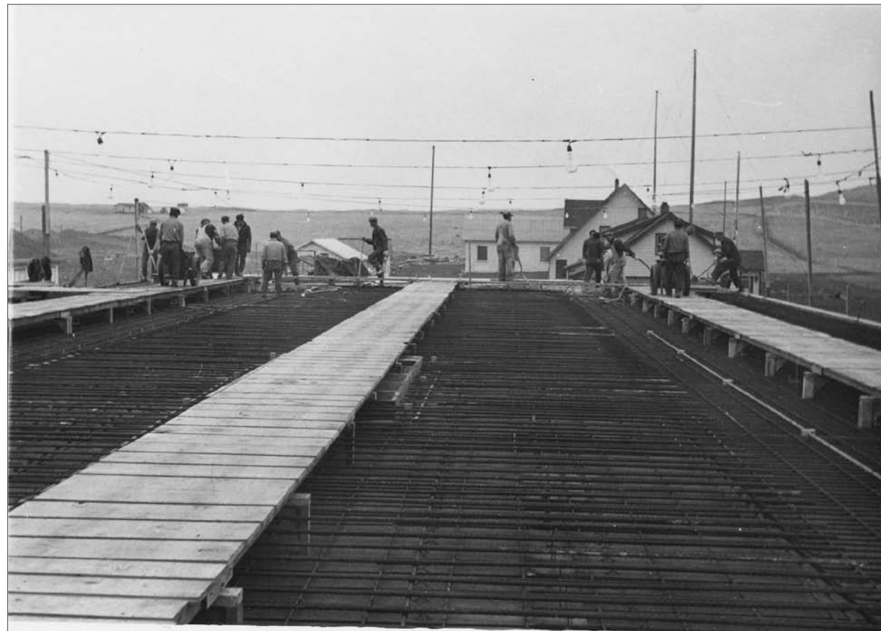
Photograph No. 95-ADMC-2090 (Photographer unknown), 1950's; Community Store/Warehouse/Laboratory under construction, looking east. Records of the National Oceanic and Atmospheric Administration, RG 370; NARA—Pacific Alaska Region (A).
