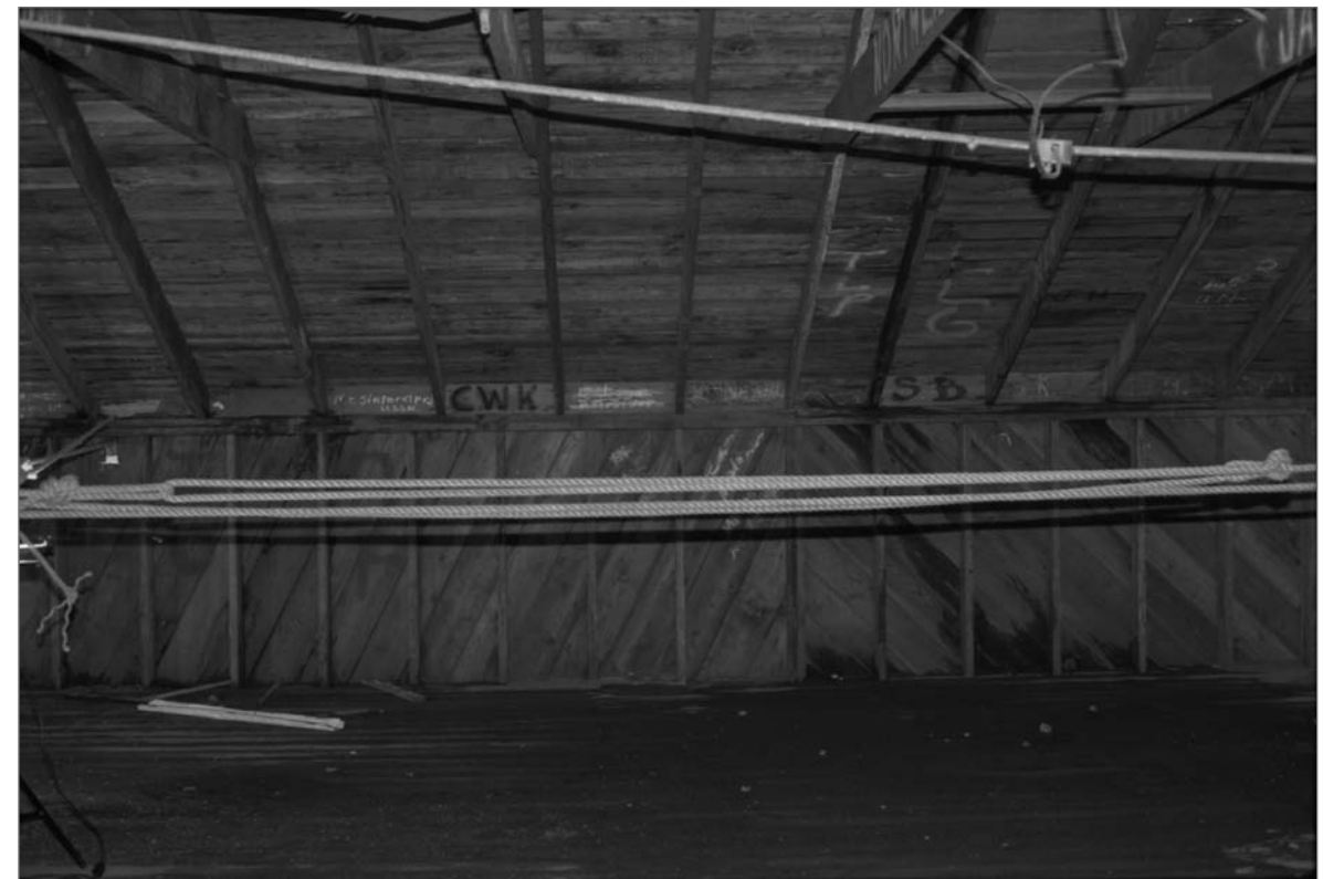
Young, Allison, photographer. 2000. Salthouse A, 2nd floor interior, west wall (north to south: left to right). Note rope linked with the building structure was used to pull the building down. Photograph (35mm). NOAA, NOS, Pribilof Project Office, Seattle: sheet JL 111379.4, neg. 4198, NMML; series includes negatives 4191 through 4202, excluding 4195.
