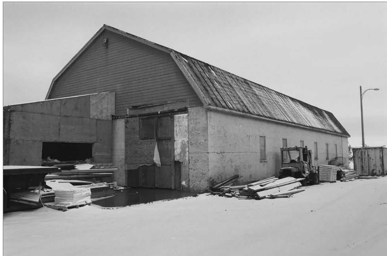
Mobley, Charles, photographer. 2007. West and north sides, Equipment Garage/Halibut Plant. Photograph (35mm) . NOAA, NOS, Pribilof Project Office, Seattle.
