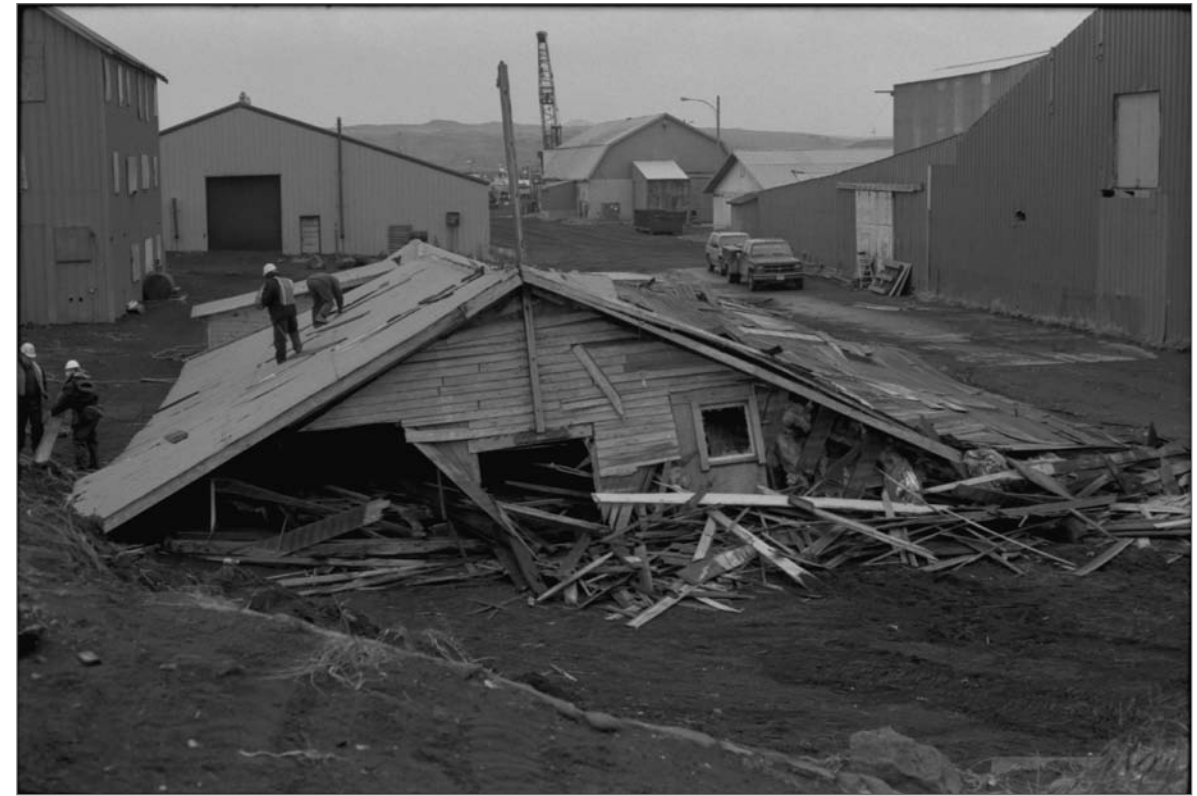
Young, Allison, photographer. 2000. Salthouse A during demolition activities looking north; Fouke Bunkhouse (left). Photograph (35mm). NOAA, NOS, Pribilof Project Office, Seattle: sheet JL 110929.1, neg. 4262.
