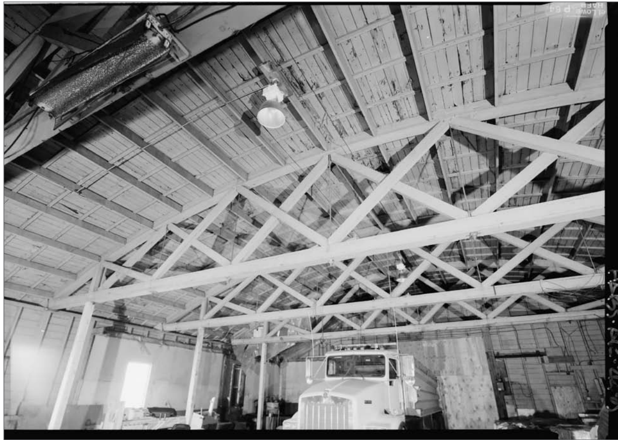
Detail of roof trusses, former Equipment Garage/Municipal Garage. Jet Lowe, photographer. Photograph (5x7). Library of Congress: HABS AK-214-9 , 2004.
