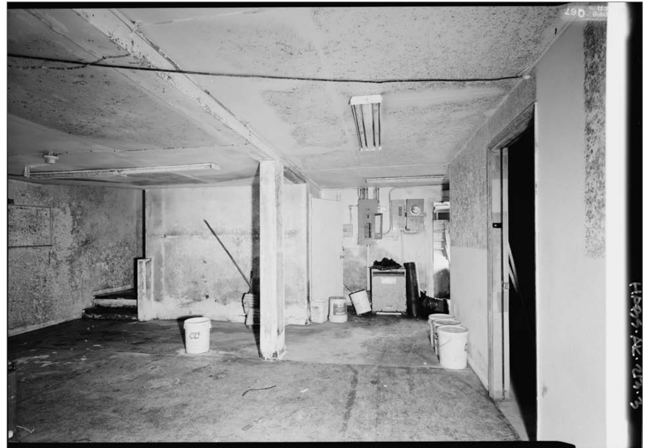
Interior, Fouke Bunkhouse. Jet Lowe, photographer. Photograph (5x7). Library of Congress: HABS AK-213, 2004.
