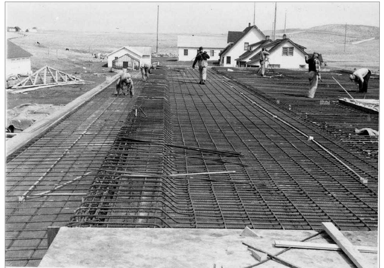
Photograph No. 95-ADMC-2085 (Photographer unknown), 1950's; Community Store/Warehouse/Laboratory under construction, looking east. Records of the National Oceanic and Atmospheric Administration, RG 370; NARA—Pacific Alaska Region (A).
