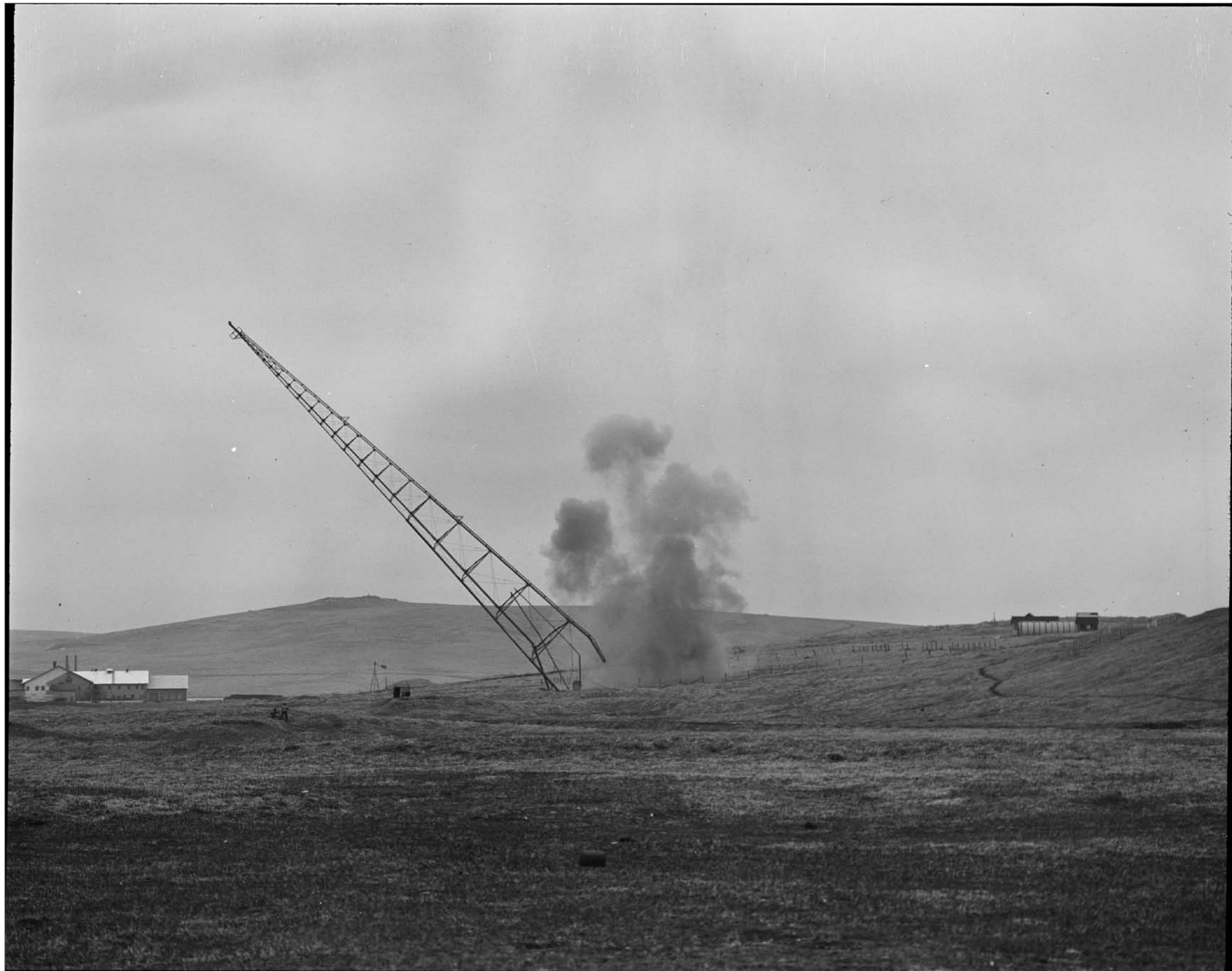
Scheffer, Victor B., photographer. June 1, 1950. According to Victor Scheffer, this is a "World War I Radio Tower being demolished by a Navy dynamiting crew." Note the By-Products Plant (background left), a windmill to the right of the plant, and a cluster of structures on the hillside. This cluster of structures has been observed in a number of photographs, but their purpose has not been identified. Photograph. NOAA, NMML Library, Seattle: Victor B. Scheffer Collection, Fur-Seal Archives, neg. no. 2750.
