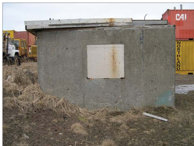
Winandy, David, photographer. 2006. Power Plant, showing east side of Saltwater Well House 3, March 3, 2006. Photograph (digital) . NOAA, NOS, Pribilof Project Office, Seattle.
