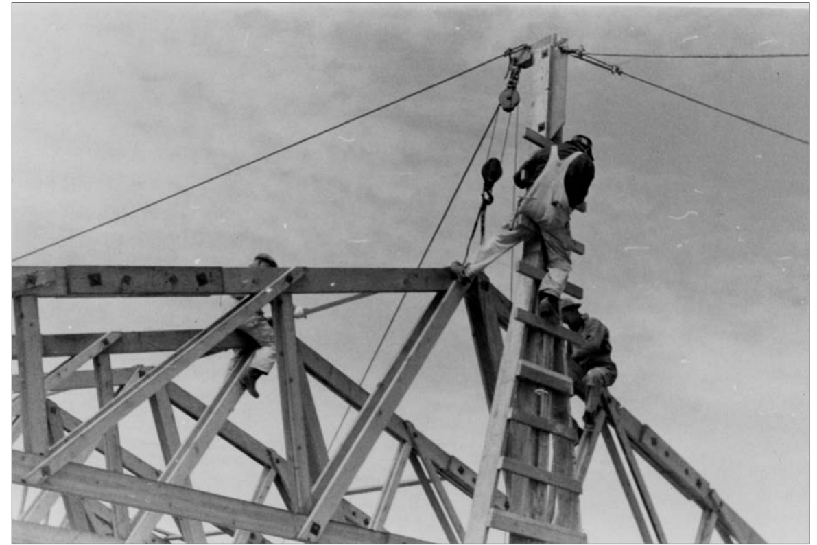
Photograph No. 95-ADMC-2011 (Photographer unknown), 1950's; Men installing trusses, Community Store/Warehouse/Laboratory. Records of the National Oceanic and Atmospheric Administration, RG 370; NARA—Pacific Alaska Region (A).
