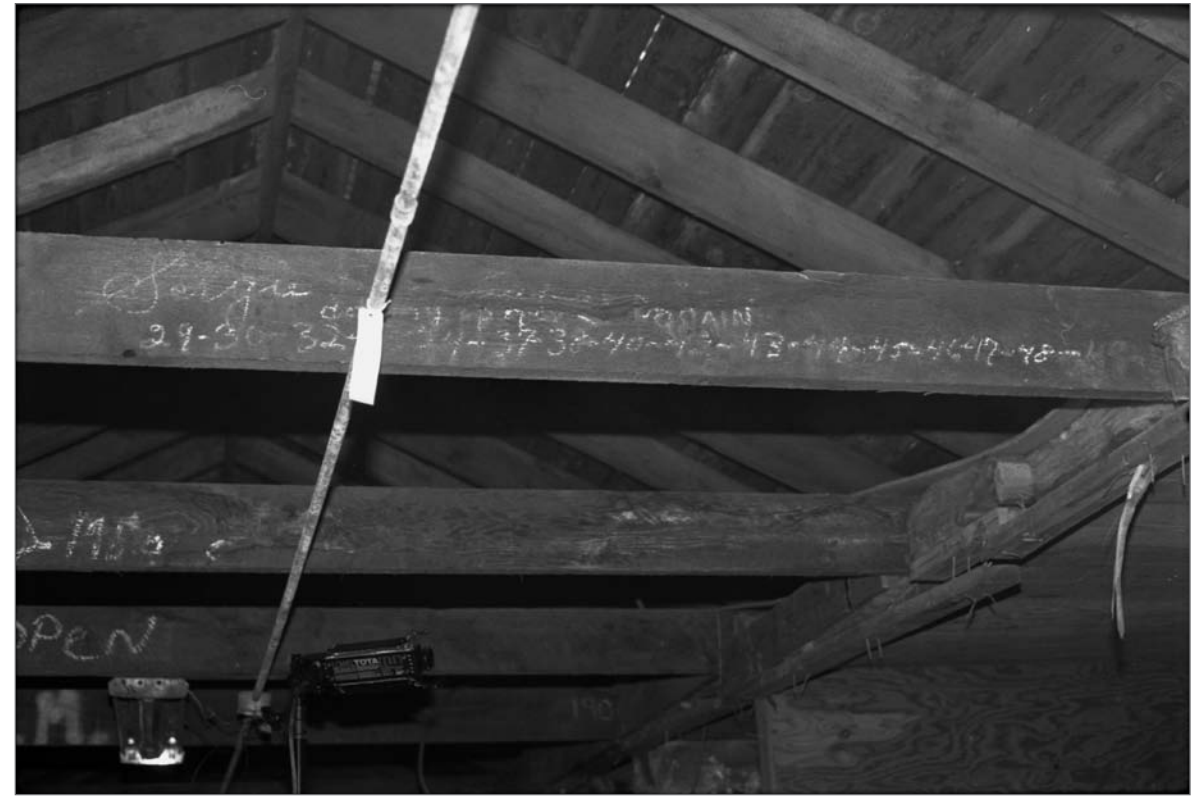
Young, Allison, photographer. 2000. Chalk, "Sergie [illegible] 29-30-32- [illegible] 34-37-38-40-42-43-44-45," on joist; electrical conduit and fluorescent light fixture running on joists, and a photographer's TOTA lamp, 2nd floor Salthouse A. Photograph (35mm). NOAA, NOS, Pribilof Project Office, Seattle: sheet JL 111379.2, neg. 4095.
