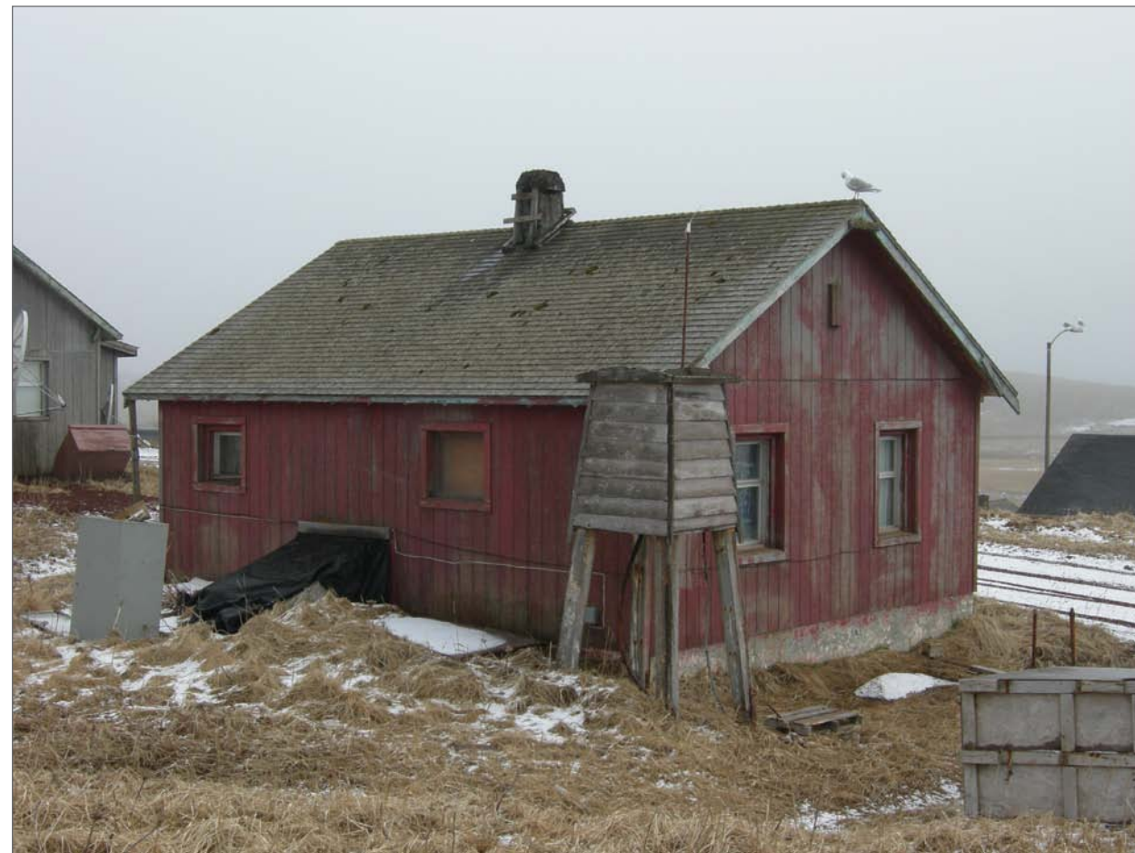
Mobley, Charles, photographer. 2007. West and south sides, Aleut Laborer House 32. Photograph (35mm). NOAA, NOS, Pribilof Project Office, Seattle.
