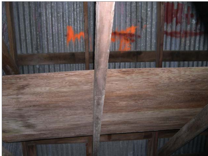
Winandy, David B., photographer. March 21, 2006. Interior, Shingle Shed. Photograph (digital). NOAA, NOS, Pribilof Project Office, Seattle.
