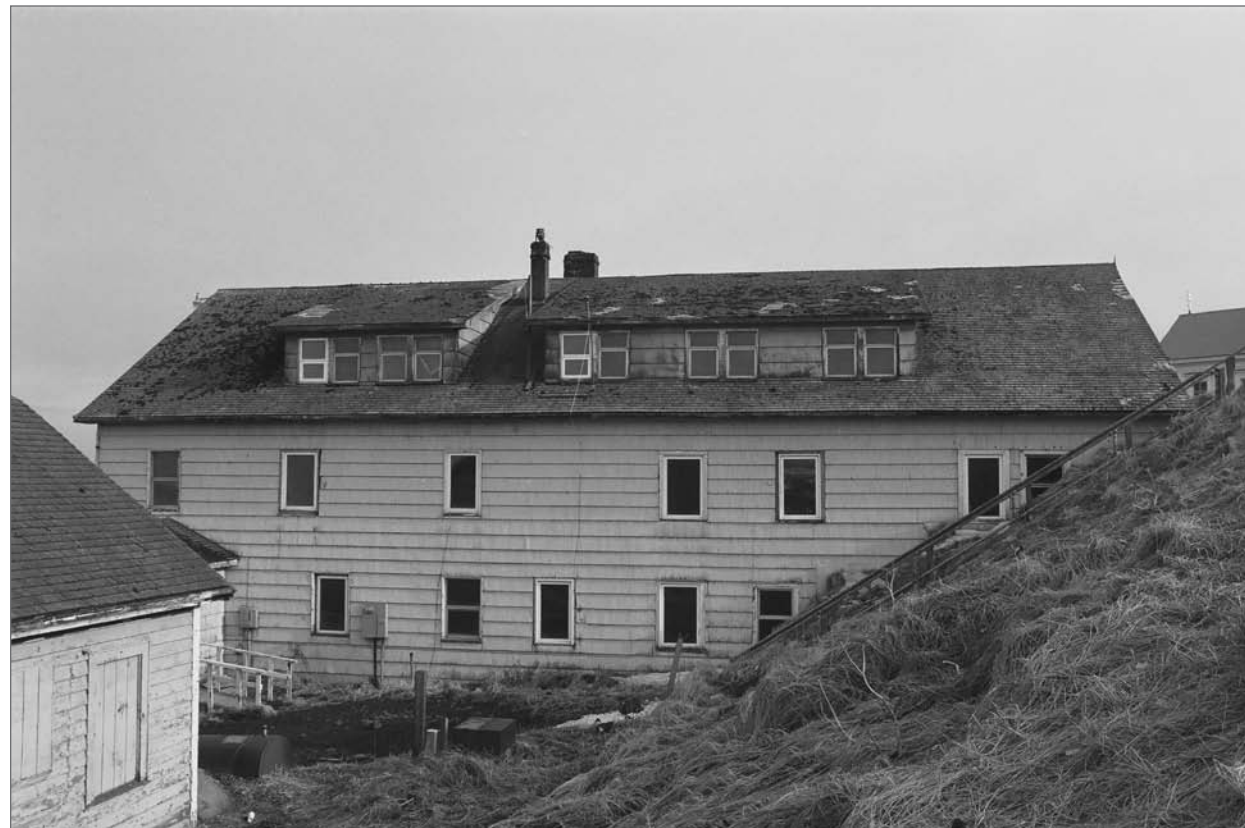
Mobley, Charles, photographer. 2007. North side, King Eider Hotel, formerly called the Company House.
