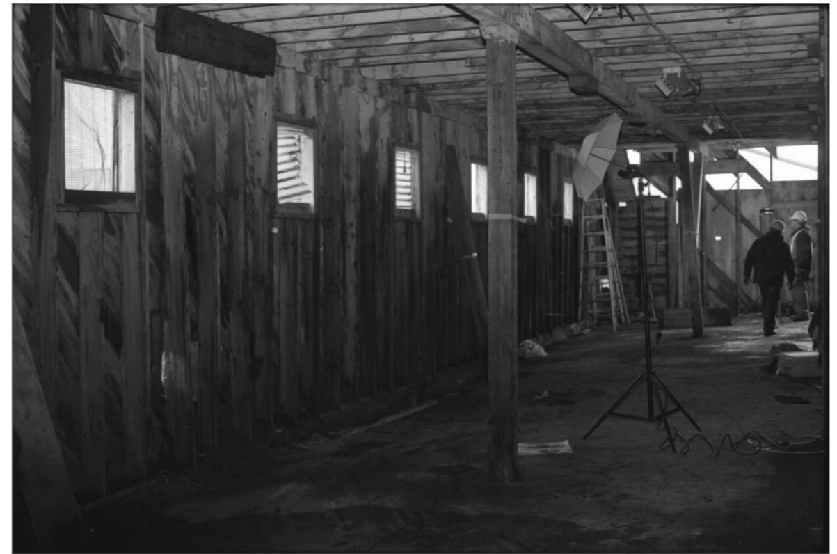
Young, Allison, photographer. 2000. Interior northwest wall, barrel chute in background, windows, wall studs, sheathing, ceiling support structures including posts, load bearing beam, floor joists, and fluorescent lighting fixtures; also light reflector (umbrella) on stand for photography and two men in background making preparations to demolish building 1st floor Salthouse A. Photograph (35mm) . NOAA, NOS, Pribilof Project Office, Seattle: sheet JL 111379.1, neg. 4015.
