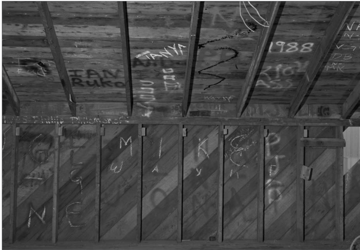
Lindsay, John A., photographer. 2000. Graffiti on wall sheathing and roof decking; second floor of Salthouse A. Photograph (6x7cm) . NOAA, NOS, Pribilof Project Office, Seattle: sheet JL110930.5, neg. 4368.
