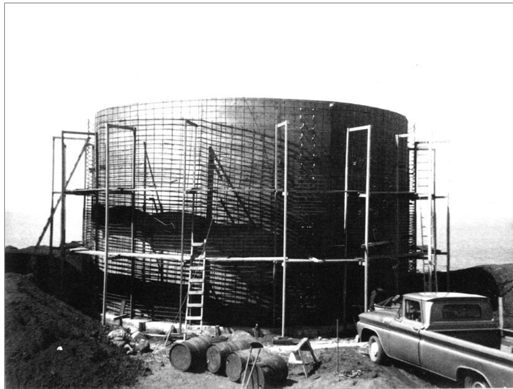
Photograph No. 95-ADMC-3026 (Photographer unknown), 1966; Water reservoir under construction on Village Hill. Records of the National Oceanic and Atmospheric Administration, RG 370; NARA—Pacific Alaska Region (A).
