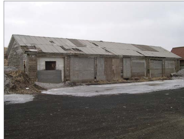
Winandy, David, photographer. 2006. West side and south front, Six-Car Garage, March 21, 2006. Photograph (digital). NOAA, NOS, Pribilof Project Office, Seattle.
