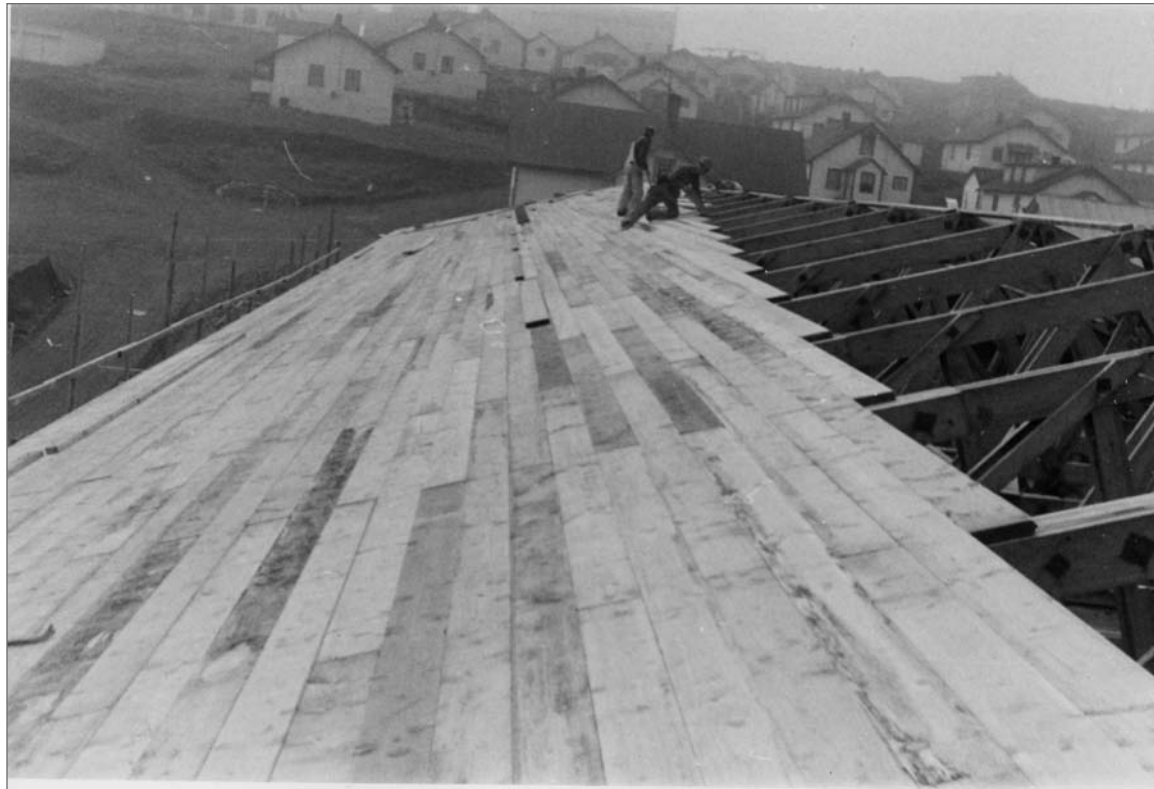
Photograph No. 95-ADMC-2006 (Photographer unknown), 1950's; Installing roof, Community Store/Warehouse/Laboratory under construction, looking west. Records of the National Oceanic and Atmospheric Administration, RG 370; NARA—Pacific Alaska Region (A).
