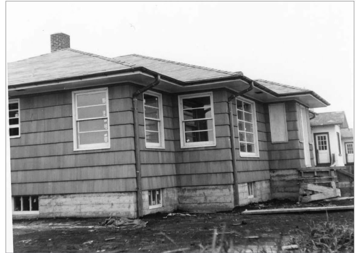
Photograph No. 95-ADMC-2509 (Photographer unknown), September 11, 1953; South and east sides, Manager's House/House 115, under construction. Records of the National Oceanic and Atmospheric Administration, RG 370; NARA—Pacific Alaska Region (A).
