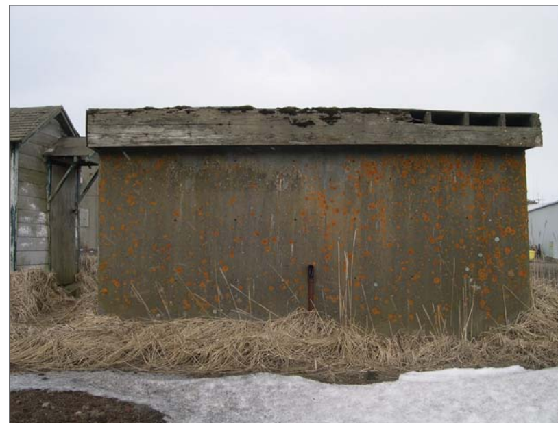
Winandy, David B., photographer. March 21, 2006. Saltwater Well House 1, March 21, 2006. Photograph (digital) . NOAA, NOS, Pribilof Project Office, Seattle.
