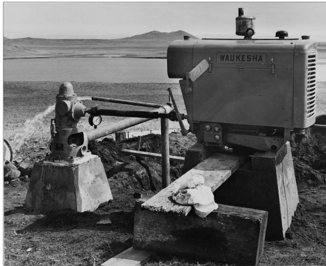
Photograph No. 95-ADMC-926 (Photographer unknown), 1956; Pump at Pumphouse (Stony) Lake. The lake supplied drinking water for the use of residents. Records of the National Oceanic and Atmospheric Administration, RG 370; NARA—Pacific Alaska Region (A).
