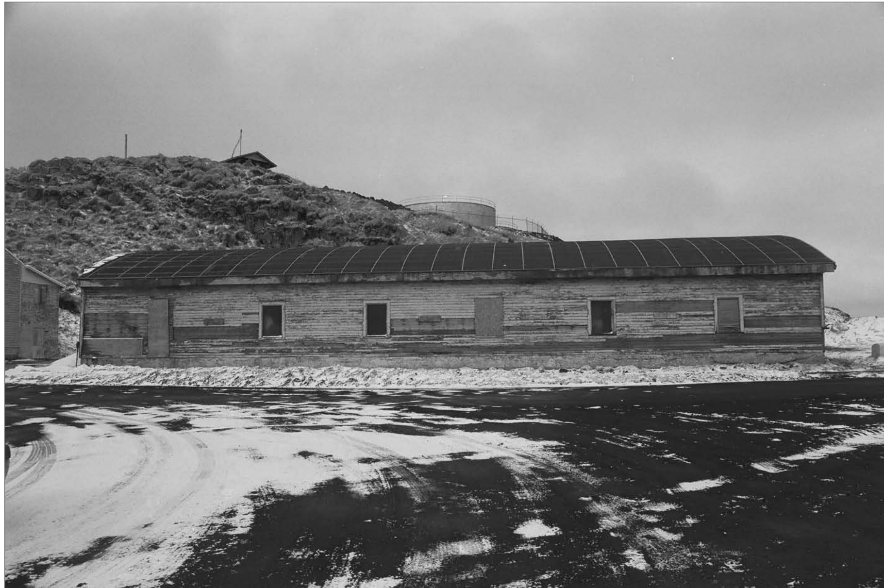
Mobley, Charles, photographer. 2007. East side, former Equipment Garage/Municipal Garage. Photograph (35mm) . NOAA, NOS, Pribilof Project Office, Seattle.
