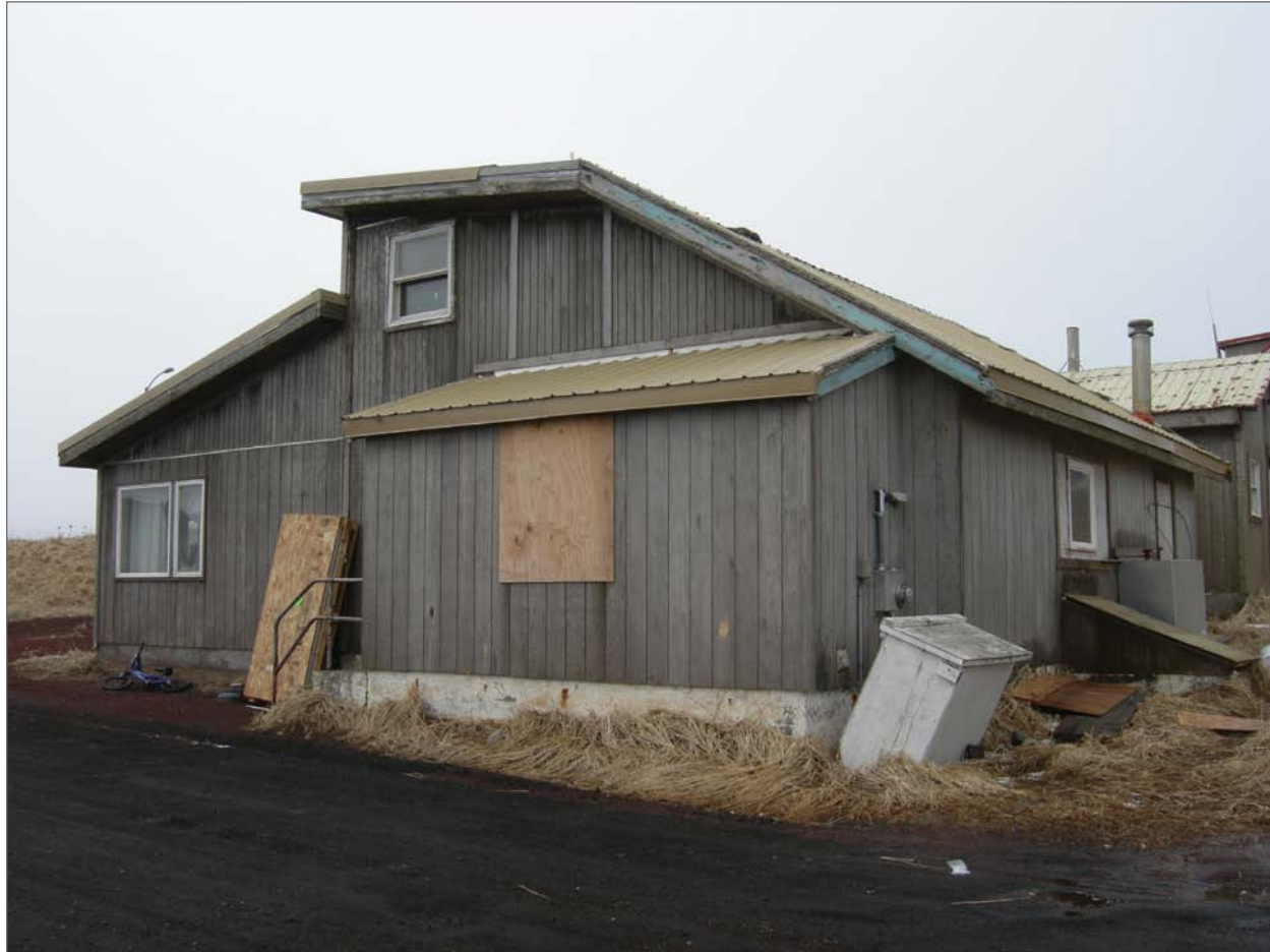
Mobley, Charles, photographer. 2007. East front and north side, Aleut Laborer House 50. Photograph (35mm). NOAA, NOS, Pribilof Project Office, Seattle.
