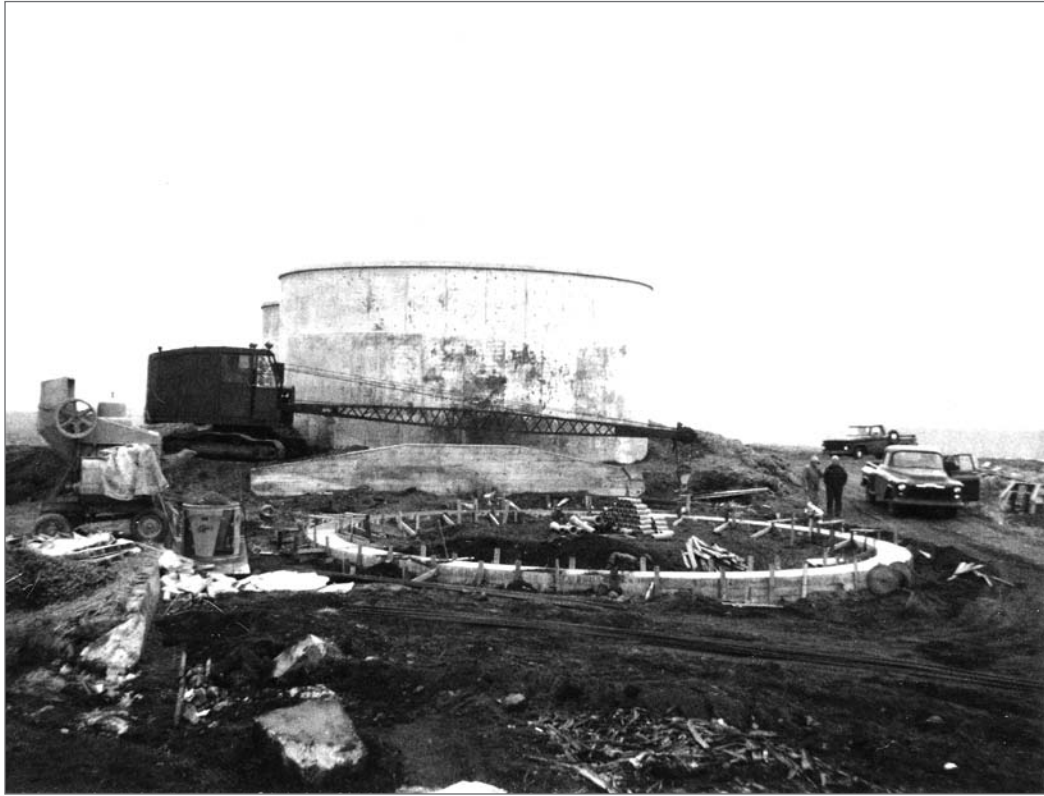
Photograph No. 95-ADMC-3024 (Photographer unknown), 1966; Water reservoir under construction on Village Hill. Records of the National Oceanic and Atmospheric Administration, RG 370; NARA—Pacific Alaska Region (A).
