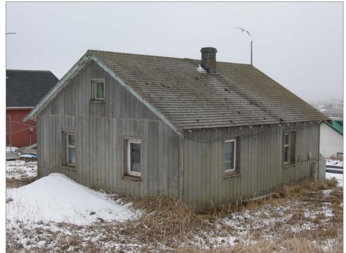
Mobley, Charles, photographer. 2007. West and south sides, Aleut Laborer House 22. Photograph (35mm). NOAA, NOS, Pribilof Project Office, Seattle.
