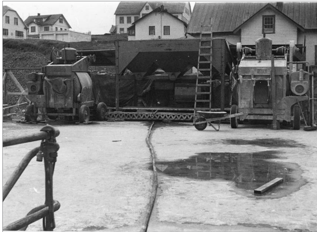
Photograph No. 95-ADMC-2088 (Photographer unknown), 1950's; Community Store/Warehouse/Laboratory under construction, looking west. Records of the National Oceanic and Atmospheric Administration, RG 370; NARA—Pacific Alaska Region (A).
