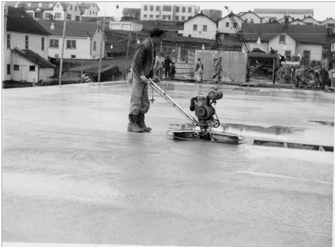
Photograph No. 95-ADMC-2086 (Photographer unknown), 1950's; Community Store/Warehouse/Laboratory under construction, looking west southwest. Records of the National Oceanic and Atmospheric Administration, RG 370; NARA—Pacific Alaska Region (A).
