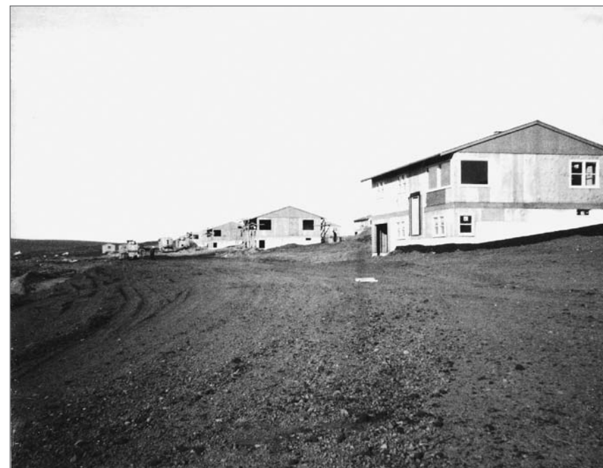
Photograph No. 95-ADMC-3022 (Photographer unknown), 1968; House under construction on Ellerman Heights. Records of the National Oceanic and Atmospheric Administration, RG 370; NARA—Pacific Alaska Region (A) .
