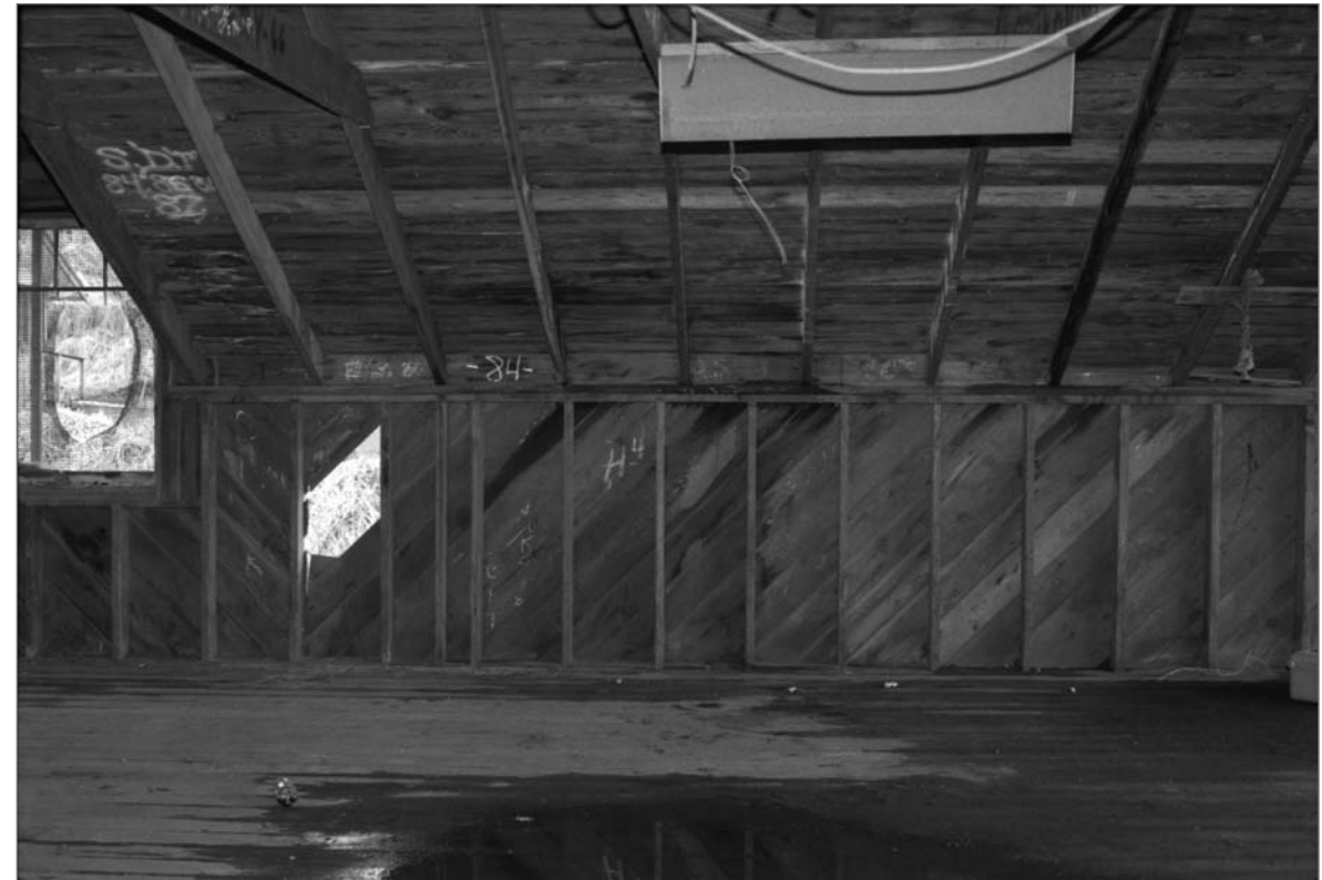
Young, Allison, photographer. 2000. Salthouse A, 2nd floor interior, west wall (north to south: left to right). Photograph (35mm). NOAA, NOS, Pribilof Project Office, Seattle: sheet JL 111379.4, neg. 4193, NMML; series includes negatives 4191 through 4202, excluding 4195.
