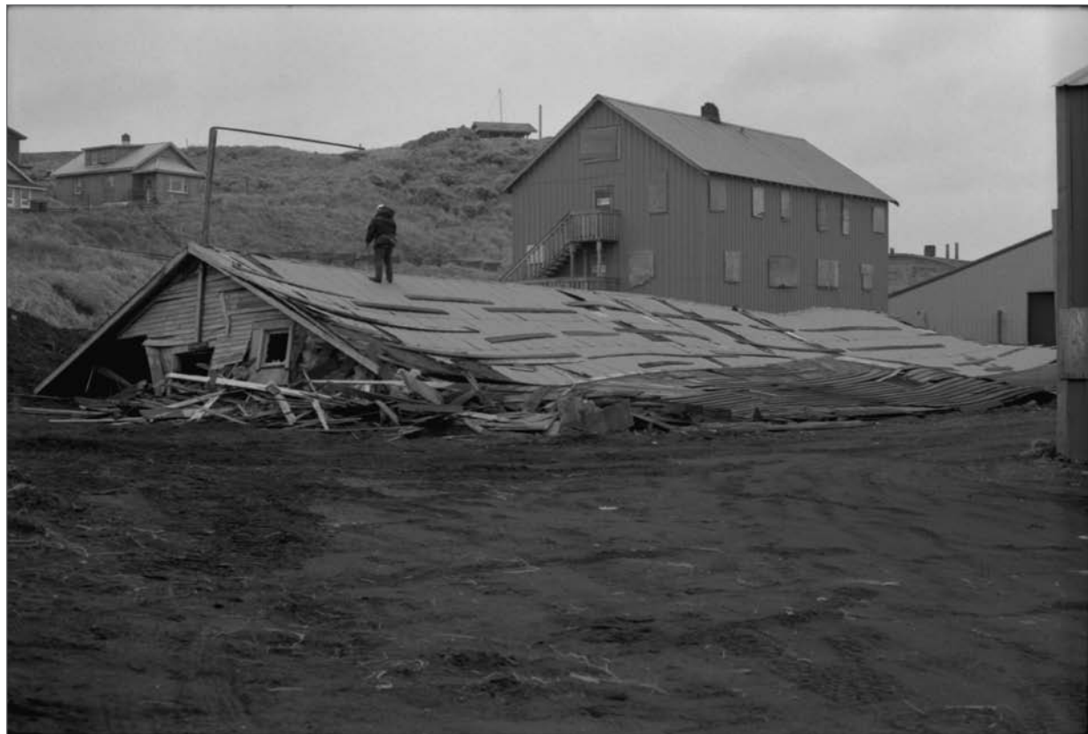
Young, Allison, photographer. 2000. Salthouse A during demolition activities looking northwest; Fouke Bunkhouse in background. Photograph (35mm). NOAA, NOS, Pribilof Project Office, Seattle: sheet JL 110929.1, neg. 4261.
