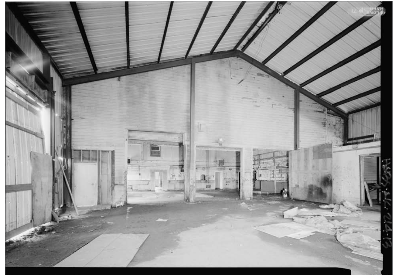
Interior, looking south, former Equipment Garage/Municipal Garage. Jet Lowe, photographer. Photograph (5x7). Library of Congress: HABS AK-214-13 , 2004.
