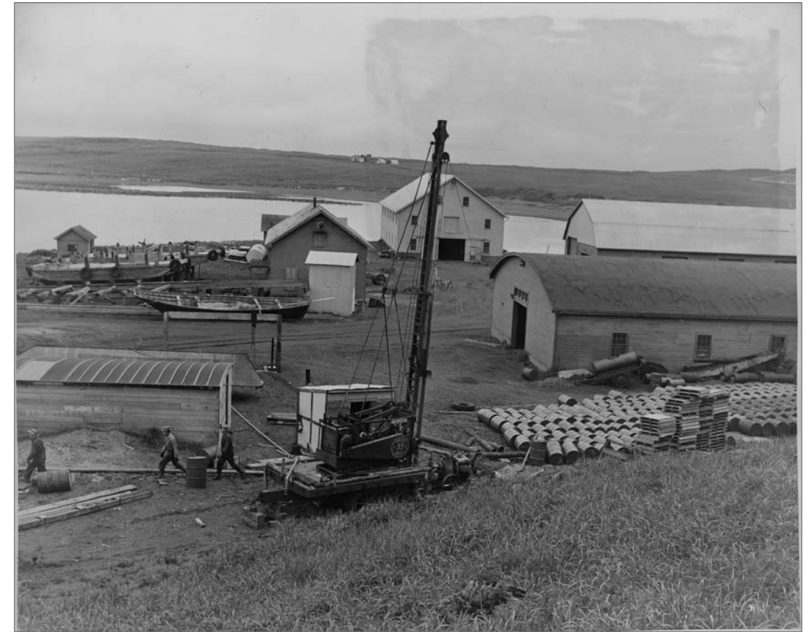
Photograph No. 95-ADMC-228 (Photographer unknown), 1955; Well drilling rig, auxiliary pump (right), and 4" pipeline discharge to bay (left). Records of the National Oceanic and Atmospheric Administration, RG 370; NARA—Pacific Alaska Region (A).
