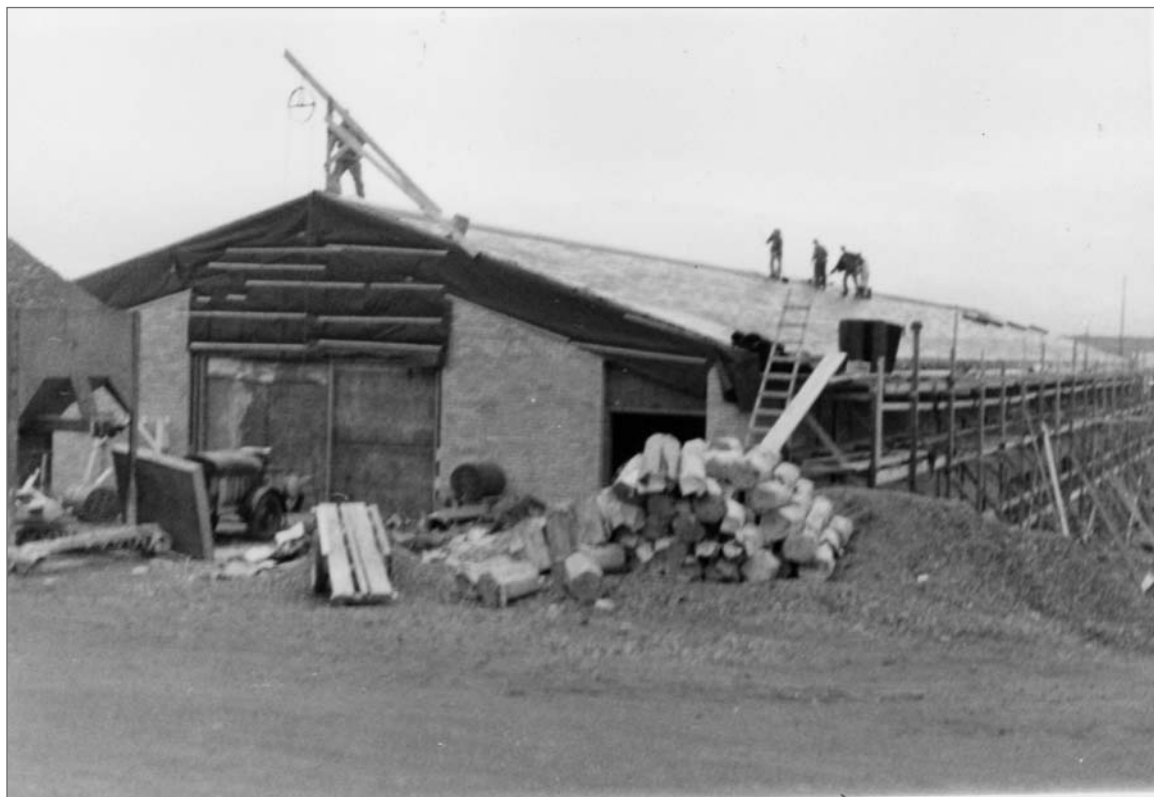
Photograph No. 95-ADMC-2003 (Photographer unknown), 1950's; Installation of roof, Community Store/Warehouse/Laboratory under construction, looking east northeast. Records of the National Oceanic and Atmospheric Administration, RG 370; NARA—Pacific Alaska Region (A).
