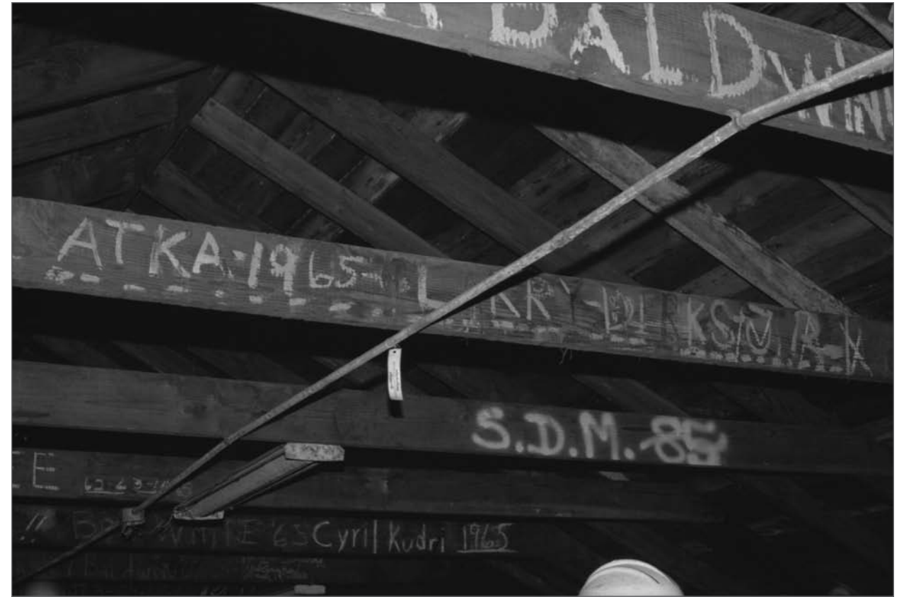
Young, Allison, photographer. 2000. Chalk on collar beams front to back "Atka 1965"; and "S.D.M. 85." Electrical conduit running north to south and fluorescent light fixture attached to joists. 2nd floor Salthouse A. Photograph (35mm). NOAA, NOS, Pribilof Project Office, Seattle: sheet JL 111379.2, neg. 4067.
