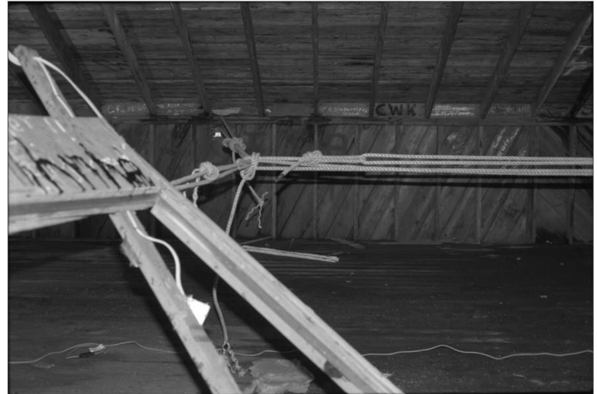
Young, Allison, photographer. 2000. Salthouse A, 2nd floor interior, west wall (north to south: left to right). Note rope linked with the building structure was used to pull the building down. Photograph (35mm). NOAA, NOS, Pribilof Project Office, Seattle: sheet JL 111379.4, neg. 4199, NMML; series includes negatives 4191 through 4202, excluding 4195.
