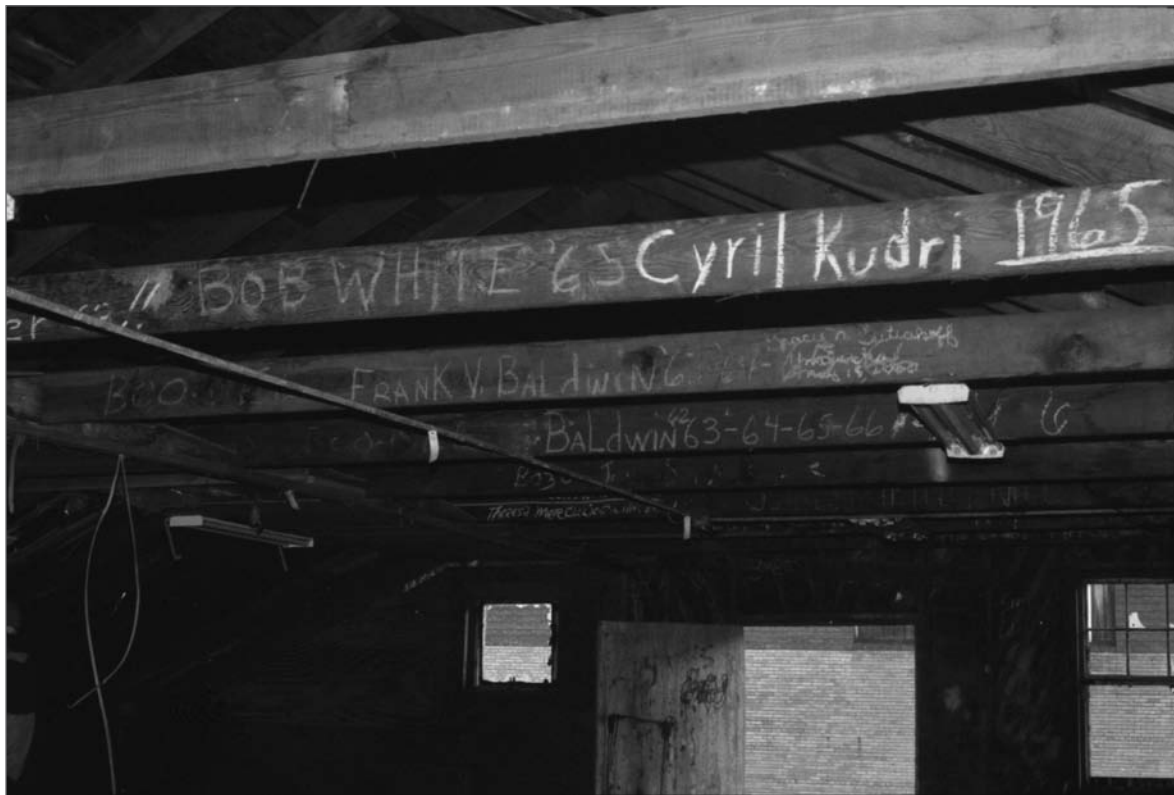
Young, Allison, photographer. 2000. Chalk on collar beams front to back "Bob White '65, Cyril Kudri 1965"; Frank V Baldwin 6 [illegible]"; and "Baldwin 62 63, 64, 65, 66 [illegible]." Electrical conduit running north to south and fluorescent light fixture attached to joists. 2nd floor Salthouse A. Photograph (35mm). NOAA, NOS, Pribilof Project Office, Seattle: sheet JL 111379.2, neg. 4099.
