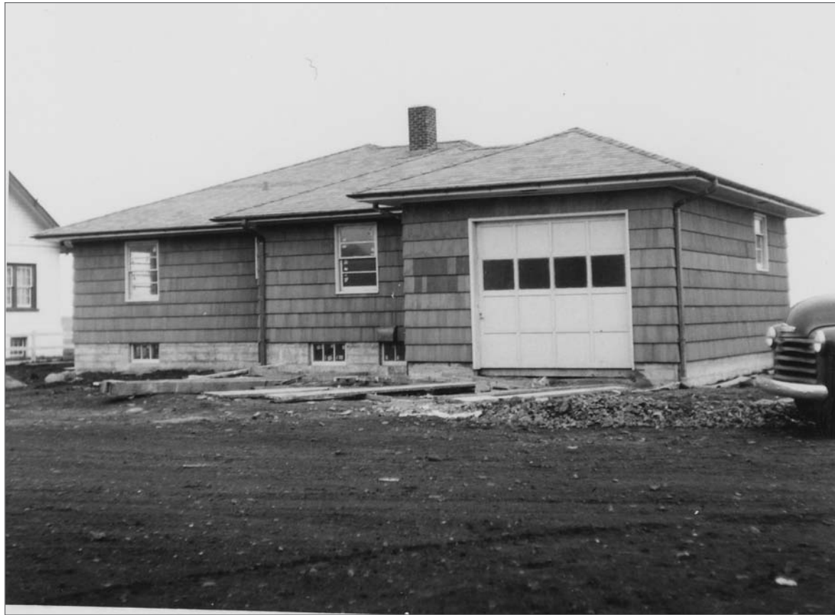
Photograph No. 95-ADMC-2508 (Photographer unknown), September 11, 1953; West front and south side, Manager's House/House 115, under construction. Records of the National Oceanic and Atmospheric Administration, RG 370; NARA—Pacific Alaska Region (A).
