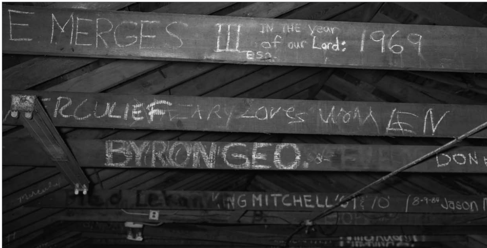
Lindsay, John A., photographer. 2000. Graffiti on ceiling rafters and cross braces; second floor of Salthouse A. Photograph (6x7cm) . NOAA, NOS, Pribilof Project Office, Seattle: JL111381.7, neg. 3883.
