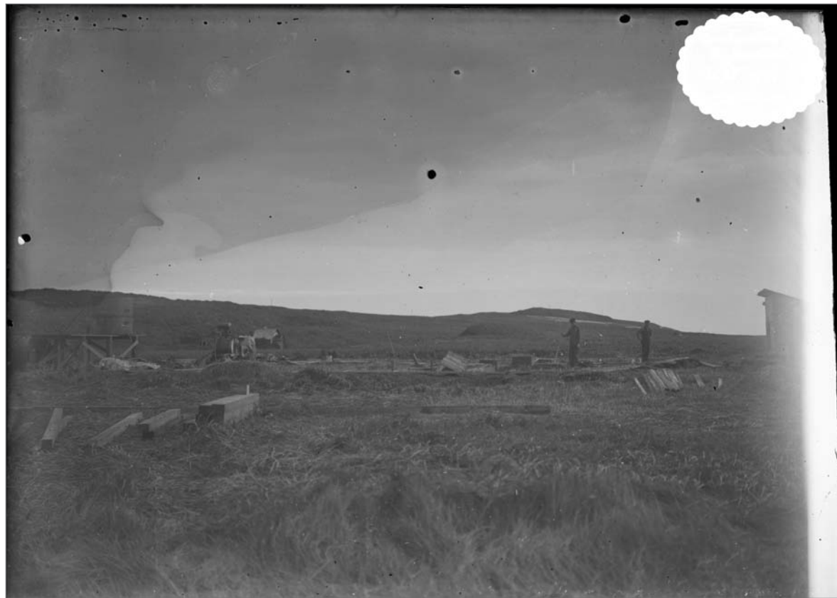
Photograph No. USBF 2.50 (Photographer G Dallas Hanna), September 1918; Construction of By-Products Plant. Records of the National Oceanic and Atmospheric Administration, RG 370; NARA—Pacific Alaska Region (A).
