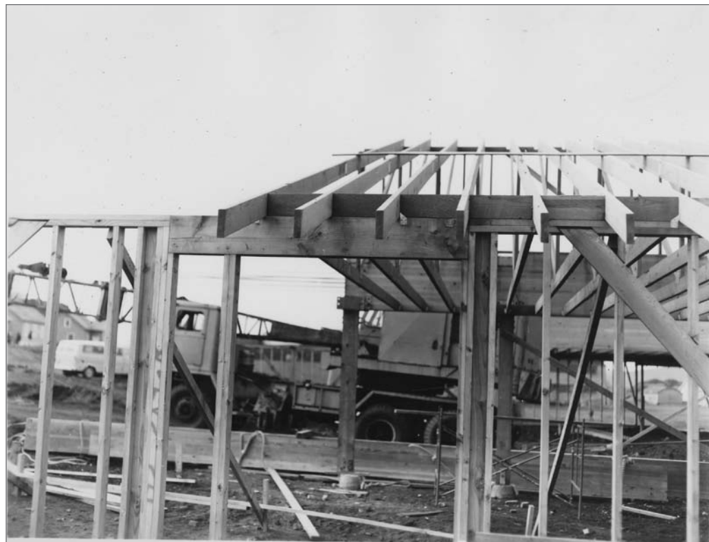
Photograph No. 95-ADMC-2168 (Photographer unknown), 1972; Construction of St. Paul Elementary and Junior High School. Records of the National Oceanic and Atmospheric Administration, RG 370; NARA—Pacific Alaska Region (A).
