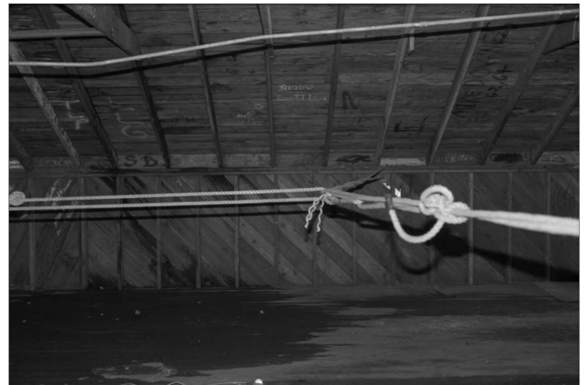
Young, Allison, photographer. 2000. Salthouse A, 2nd floor interior, west wall (north to south: left to right). Note rope linked with the building structure was used to pull the building down. Photograph (35mm). NOAA, NOS, Pribilof Project Office, Seattle: sheet JL 111379.4, neg. 4197, NMML; series includes negatives 4191 through 4202, excluding 4195.
