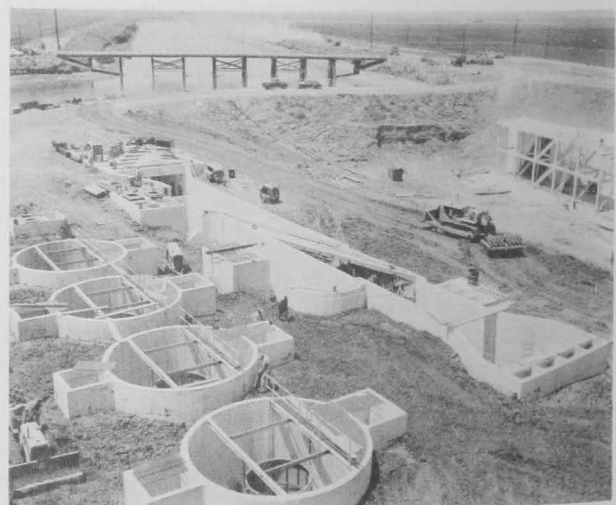
Fig. 3 - General view of construction of holding tanks, secondary louver, and pumping plant areas for the Tracy Pumping Plant on the Delta-Mendota Canal in Central California.
