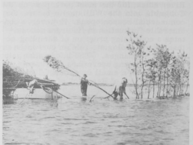
Fig. 2 - Putting in small trees for the shore leader. Using a water jet, driven by a small gasoline-powered pump on the skiff at left, a hole is dug 4 feet deep in the sand and the trees inserted 2 feet apart.
