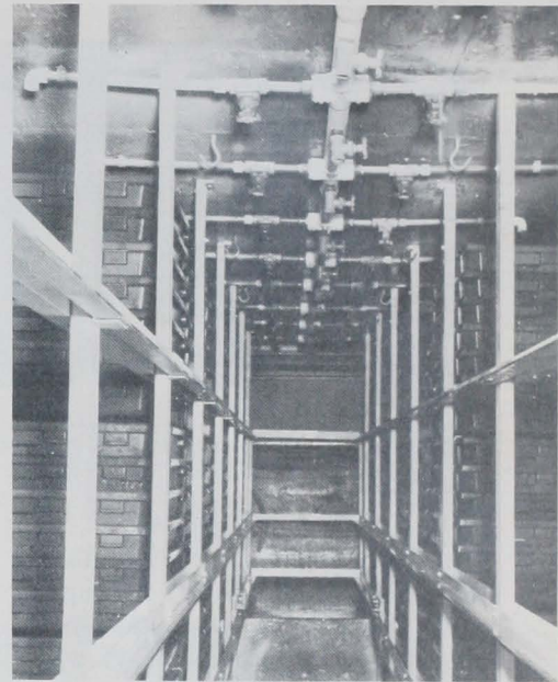
Figure 5. (above)—Arrangement of PVC distributor pipes (top, center) feeding chilled seawater to trays loaded with crabs.
